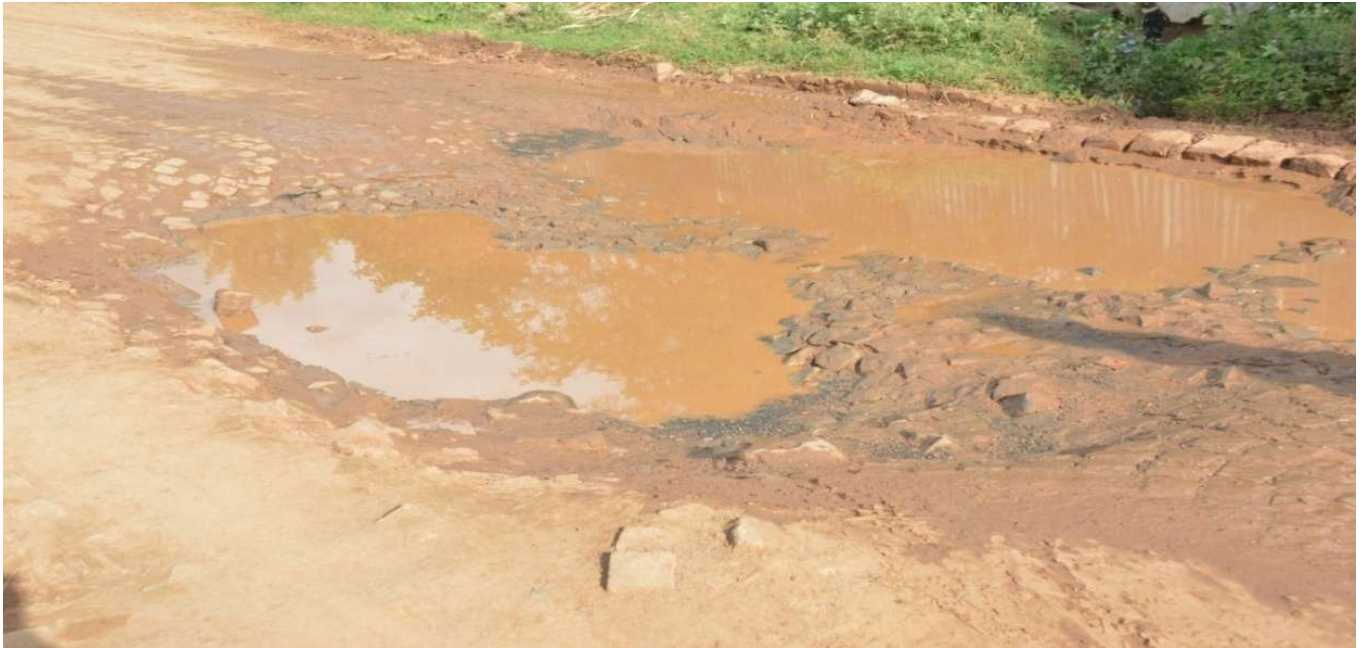
Figure 6. Deteriorated cobblestone roads by heavy vehicle
