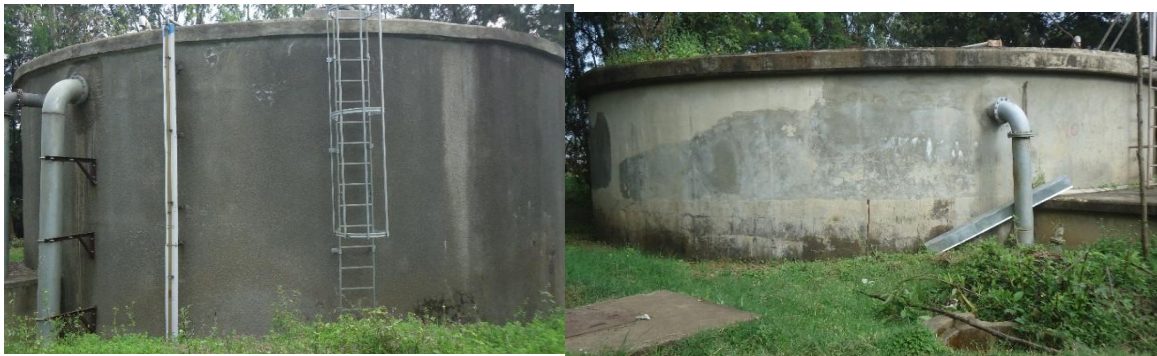
Figure 3.2 Clear water reservoir
