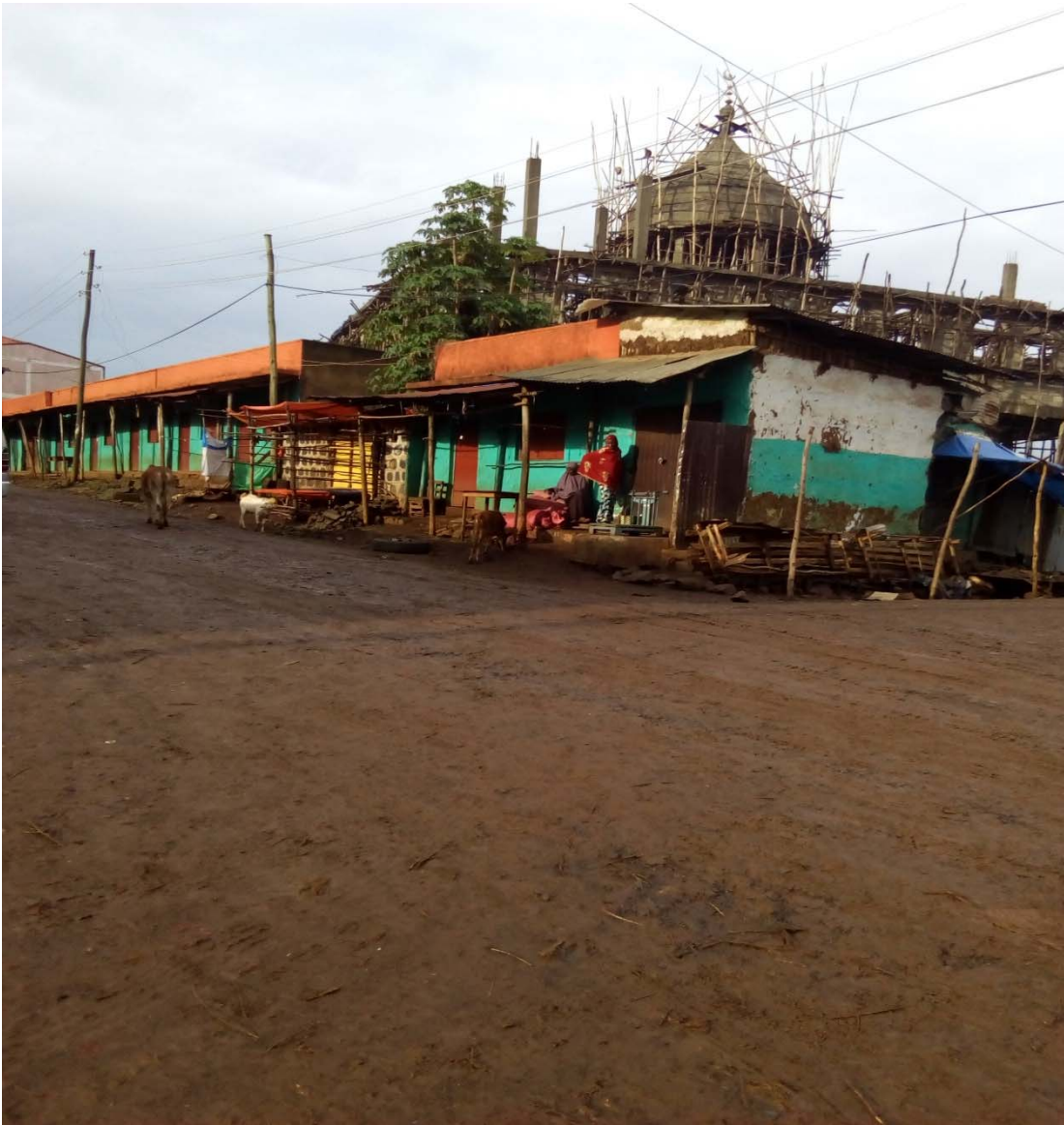
Figure 6. The new Selam mosque which is in the process of building to replace the old.
