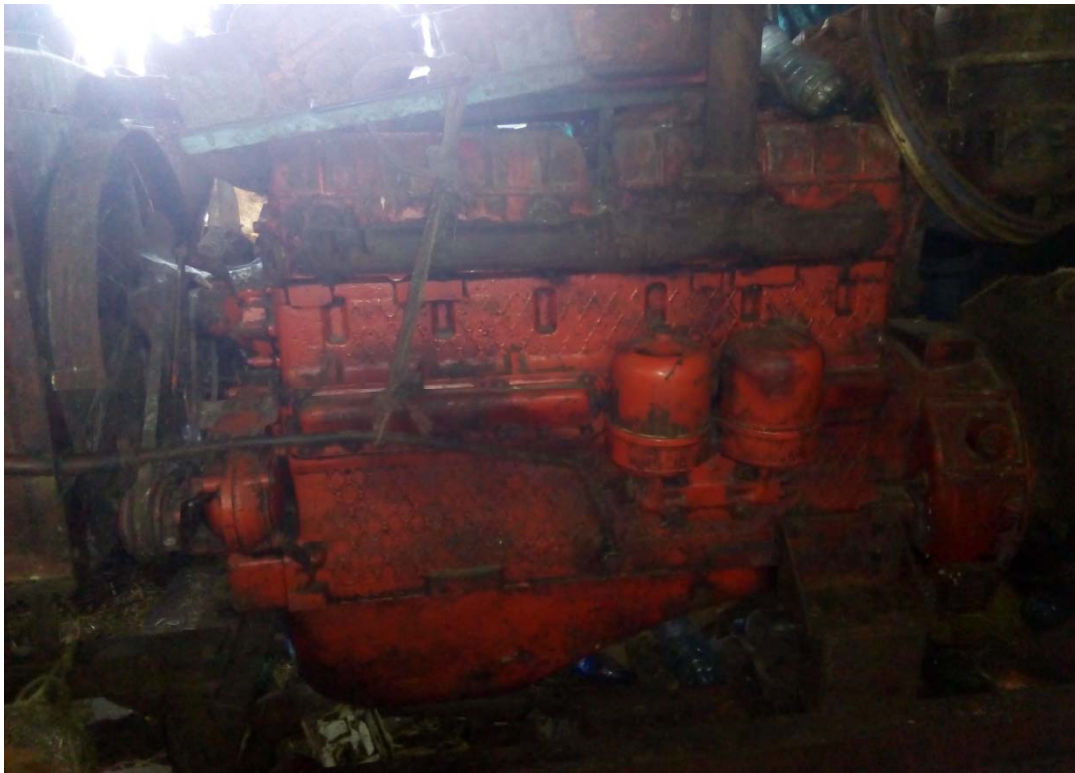
Picture 12. The first diesel engine power generator of Cooraa district
