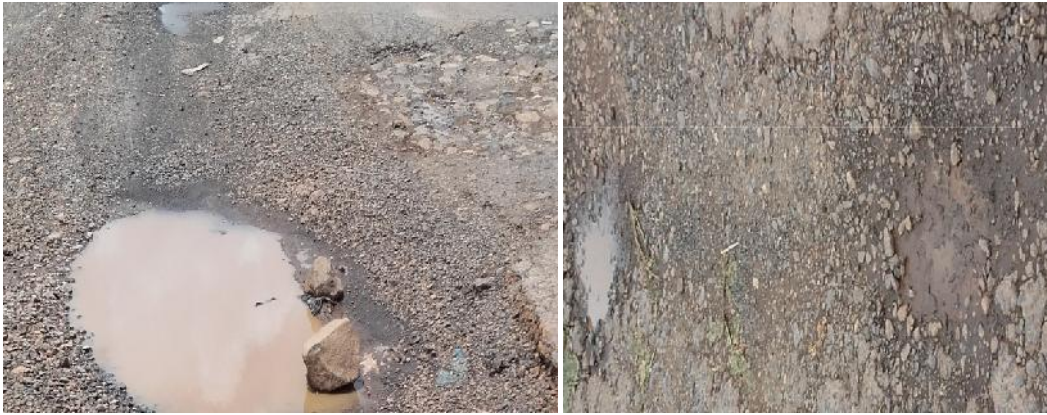
Figure 4. 9 Patching Distress type ,high Severity level Chainage 40+236
