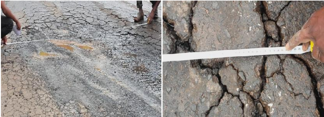
Figure 4. 2 Fatigue crack distress type and fatigue crack Distress type high severity level ,Chainage 17+670 moderate severity level, chainage 30+00
