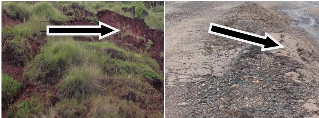
Figure 4. 12 Deformation of pavement , high Severity Levels, chainage 17+870
