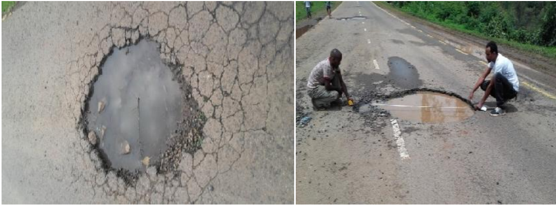
. Figure 4. 6 Potholes Distress type, high severity level ,Chainage 25+800 and Potholes distress type, high severity level, Chain age 25+100 Most of Dembi-Bedele defects are potholes
