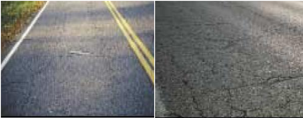
Figure 4. 3 Wheel paths Distress type, Low severity level,Chainage 46+700 and Block crack distress type ,high severity level, change 42+100
