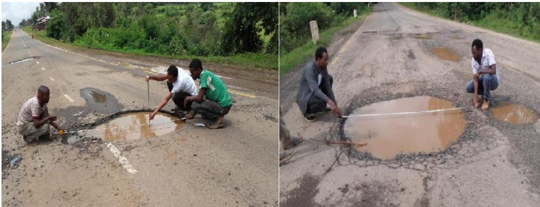
Figure 4. 7 Potholes Distress type, high severity level, Chainage 34+200 and Potholes distress type ,high severity level, Chainage 32+00
