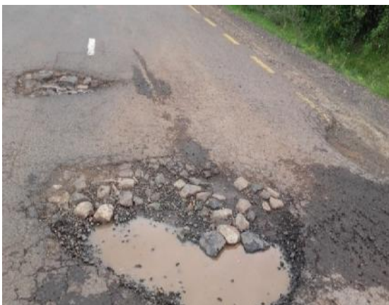
Figure 4. 4 Patch Distress type, high severity level Chainage 28+900
