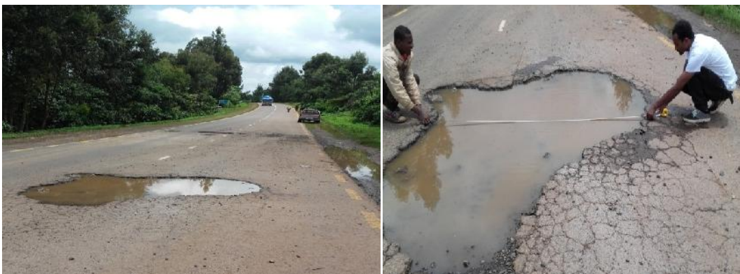
Figure 4. 8 Potholes Distress type, high Severity level, Chainage 28+200
