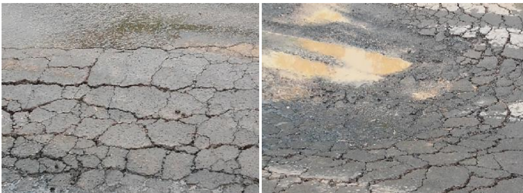
Figure 4. 1 Fatigue crack distress type, high severity level, Chainage 29+450 and fatigue crack distress type, high severity level, Chainage 29+00
