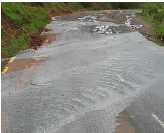
Figure 4. 11 Water in Ruts Distress Type, High Severity level, Chainage 18+850
