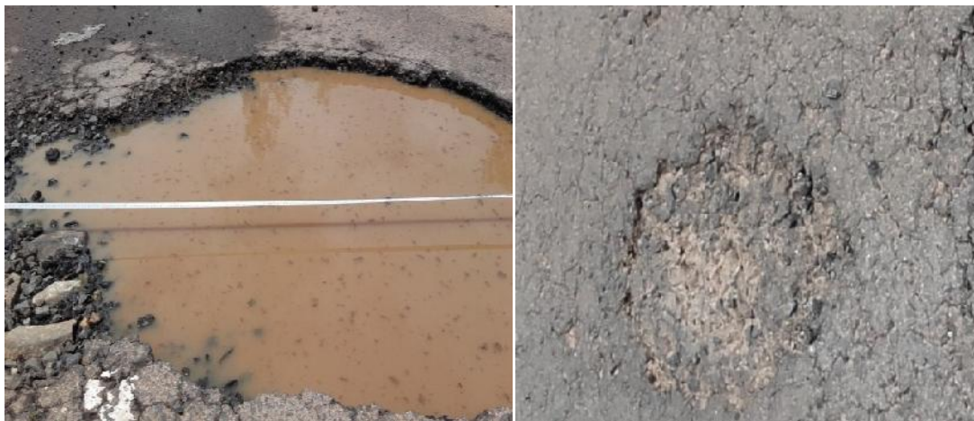
Figure 4. 5 Potholes distress type, high severity level, Chainage 19+300 and Potholes distress type Low Severity level, Chainage 26+00
