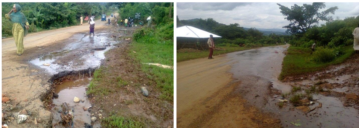
Figure 4.13 Over flooding of water on the road by poor drainage.
