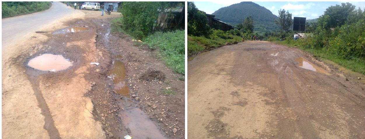
Figure 4.10 Potholes and water detention
