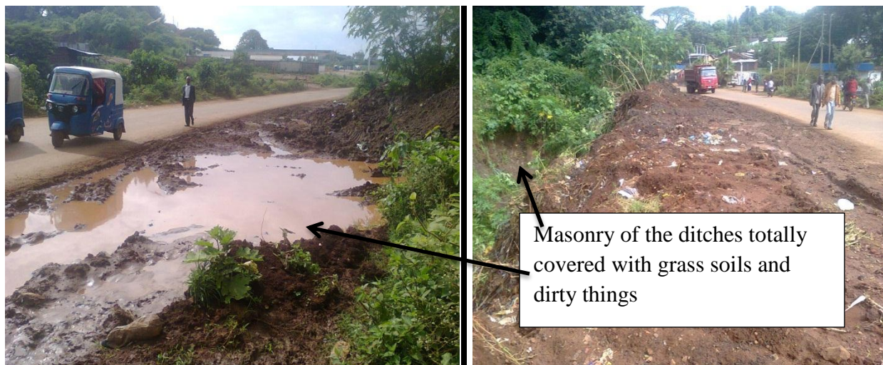
Figure.4.11 The drain blocked with silt and sand accumulation, debris and vegetation as shown.
