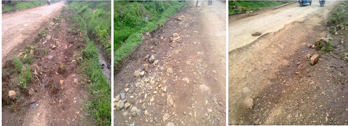
Figure 4.14 Erosion of the asphalts and shoulders by poor drainages
