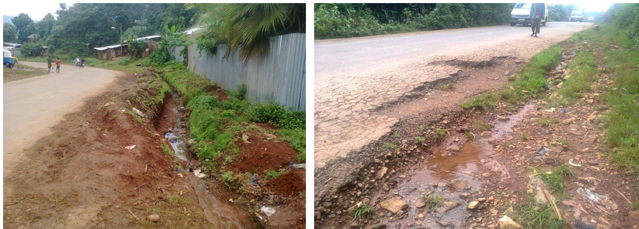
Figure 4.8 Accumulation of soils on the road and Edge of the road erosion
