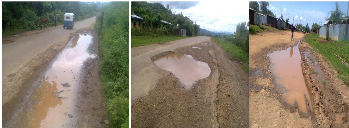
Figure 4.15 Severe failures of road edges due to water ponding on surface of road.
