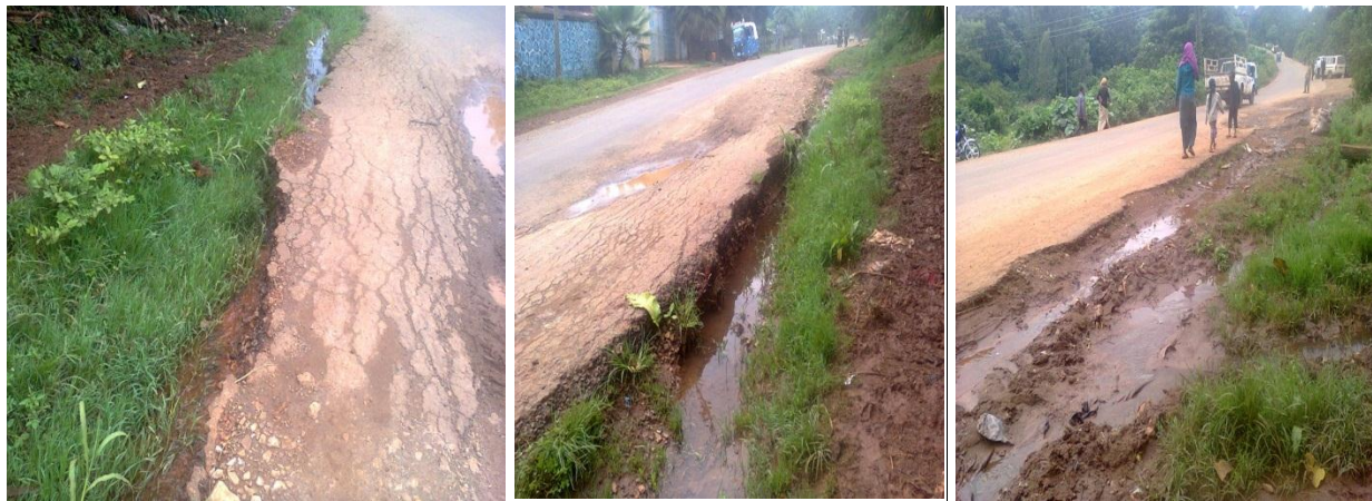
Figure 4.12 Formation of pavement cracking and edge erosion due to Poor Drainage.
