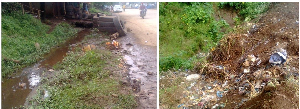
Figure 4.9 The side drain was blocked with soil, debris, vegetation, wheel and solid waste.
