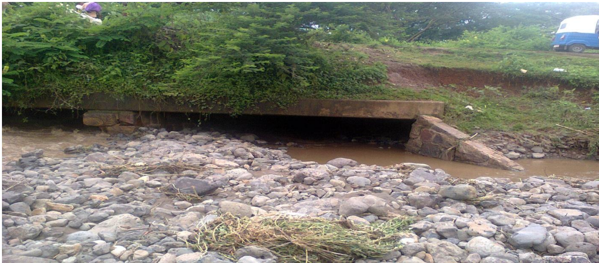
Figure 3.2 Damaged Culverts at Station 18+160
