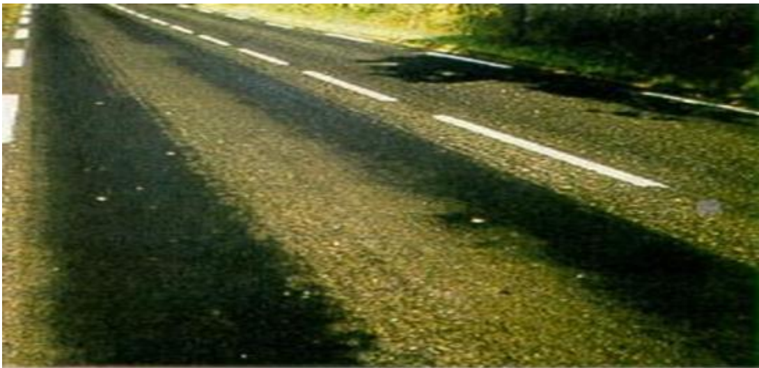
Figure 2.7 High severities raveling of asphalt surface
