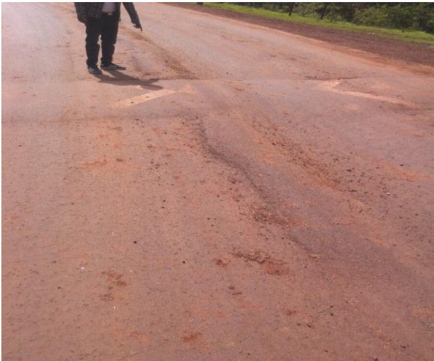
Rutting at wheel path type
