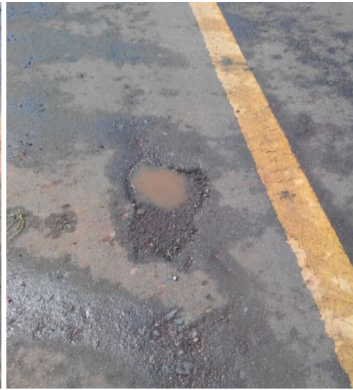
Potholes at section 2(photo10, 6, 2016)
