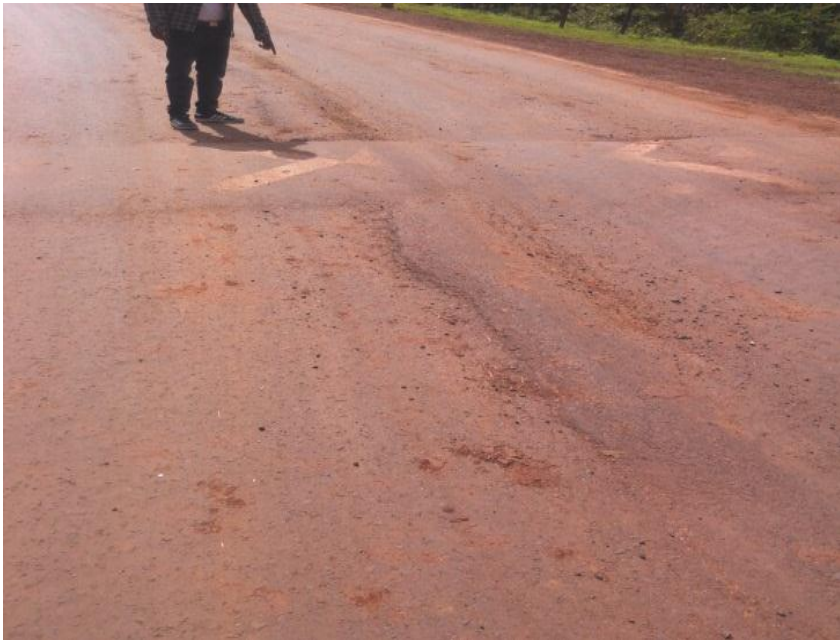
Rutting at wheel path at section 2 (photo10, 6,2016)
