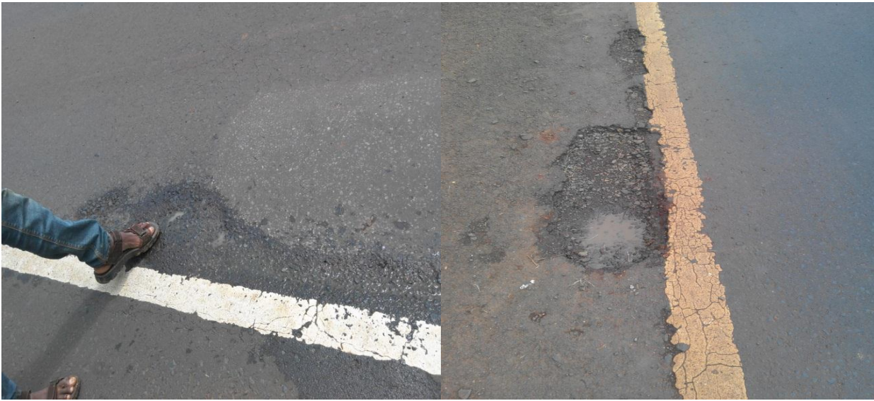
Pumping types of deterioration
