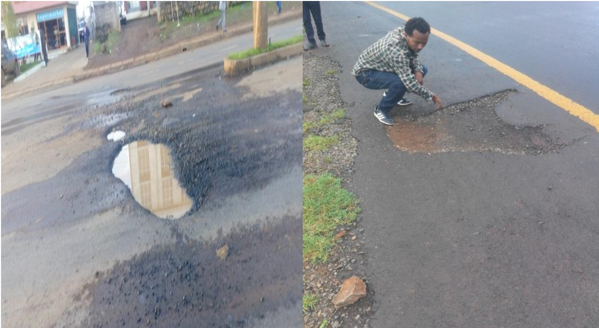
Potholes at section 1 (photo 3 ,6, 2016)
