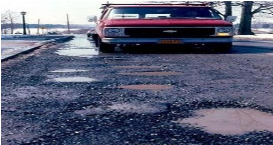
Figure 2.6 Potholes caused by poor drainage
