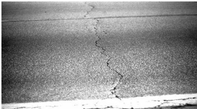
Figure 2.3 Low severity transverse cracking
