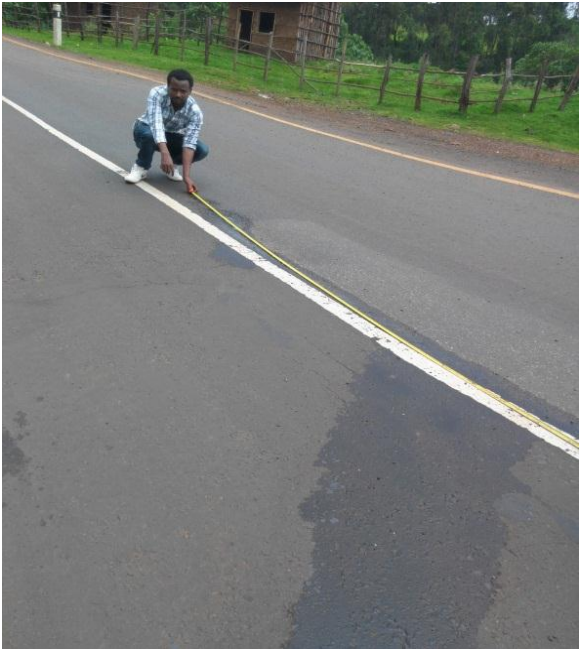
Pumping types of deterioration
