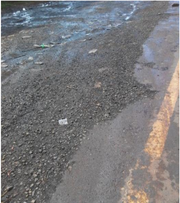
Edge cracking type of deterioration
