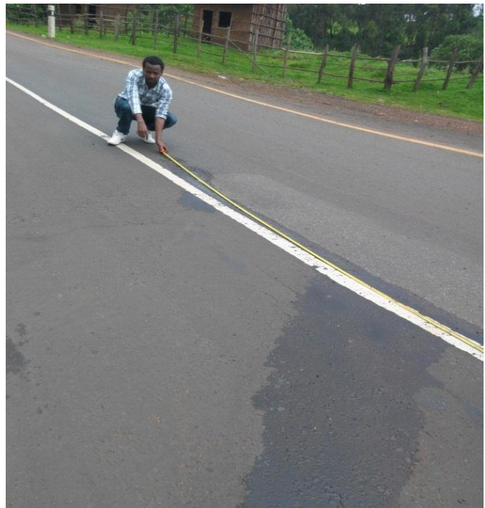
pumping type at section 1(photo 12, 6, 2016)
