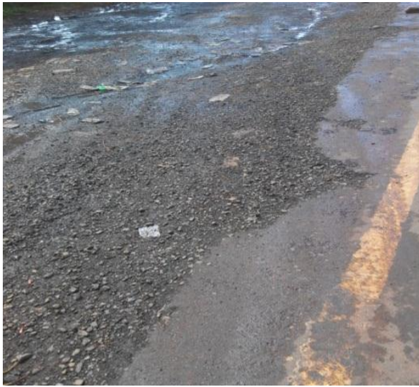
Edge cracking at section 3 (photo 15, 6, 2016)
