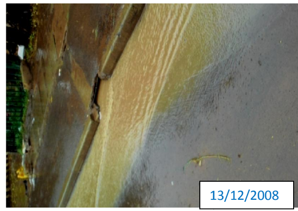
Figure-23 Inlet problem
