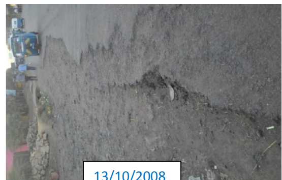
Figure-16 pavement edge raviling
