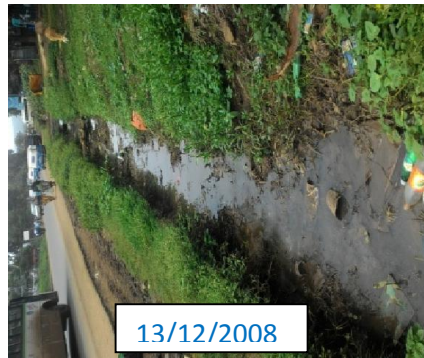
Figure-10 Drainage filled with wastes
