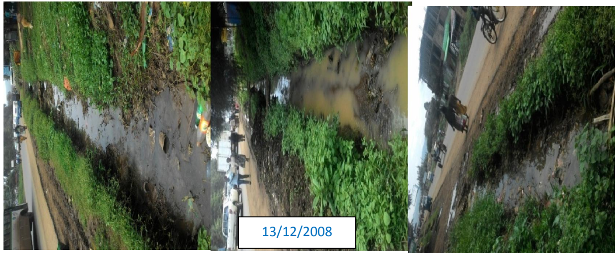
Figure-24 Drainage filled by wastes and covered by plants
