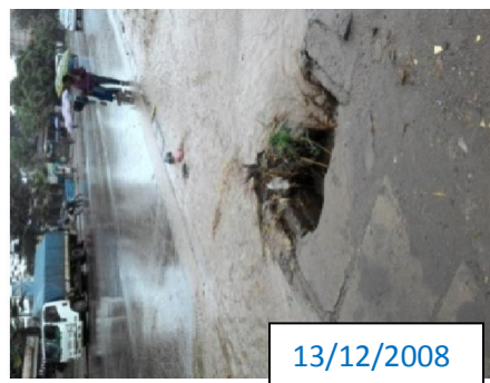
Figure-20 Failure of manhole
