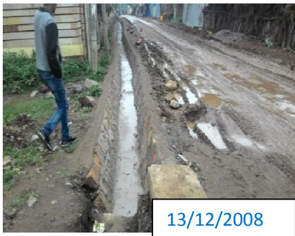
Figure- 19 Poor maintenance
