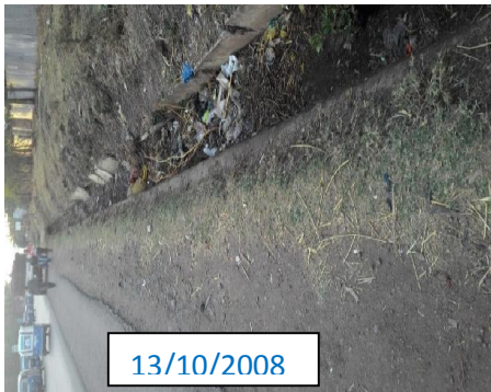
Figure-9 Drainage side failure
