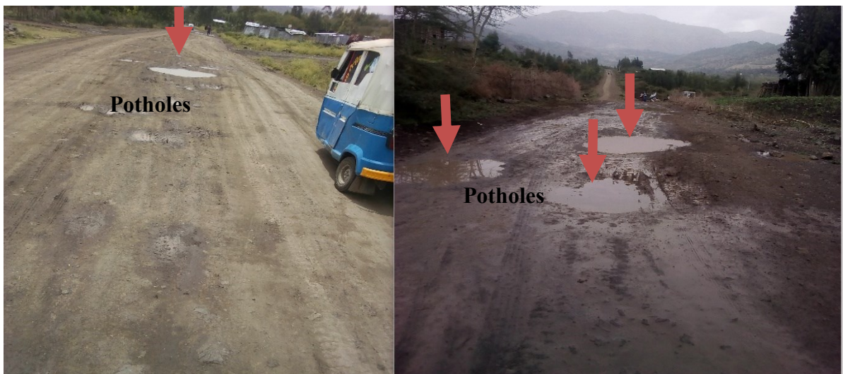
Figure 4.19 Formations of potholes and corrugation by lack of adequate crown
