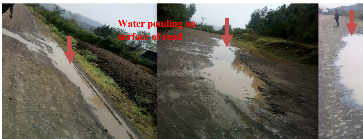
Figure 4.18 Failures of road edges due to water ponding on surface of road.
