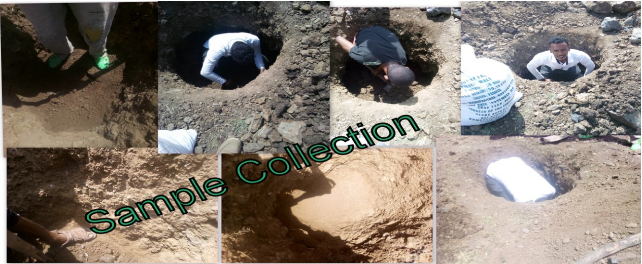
Figure 3.3 Photos of test pit taking for subgrade soil and gravel material at different stations
