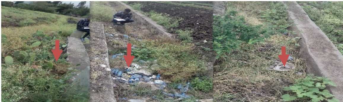
Figure 4.17 Side drain is blocked with debris, vegetation and solid waste.
