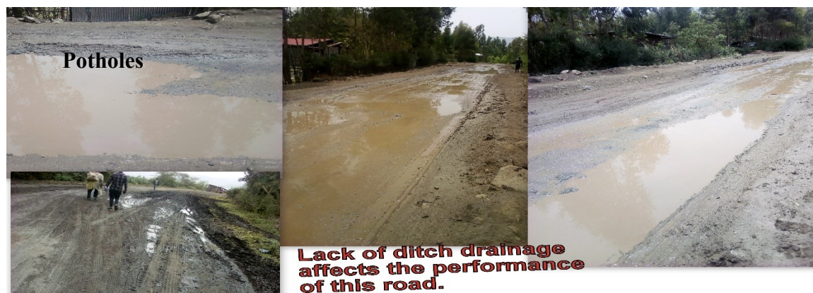
Figure 4. 22 Lack of side ditch drainage affects the performance of the road
