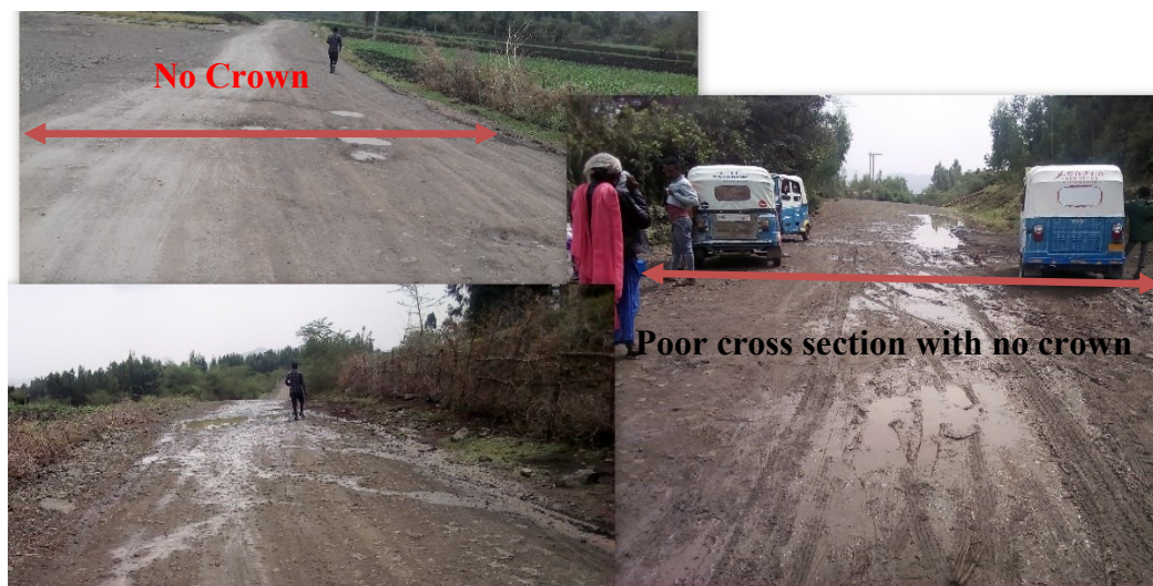
Figure 4. 20 A poor cross section with no crown on the surface of the road
