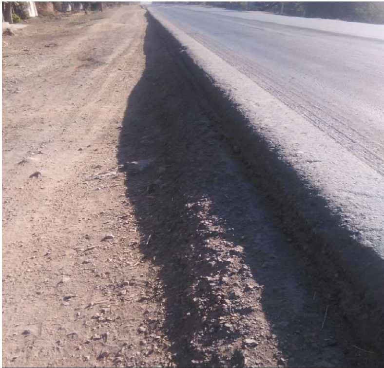
Figure4. 9 Photo shows the damaged shoulder and edge of road segment
