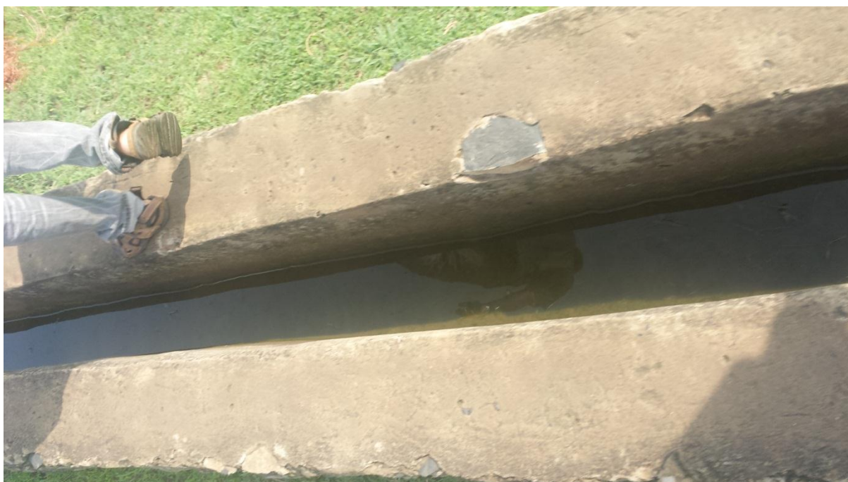
Figure: 4.8 Stagnation of water at the canal (tankua)
