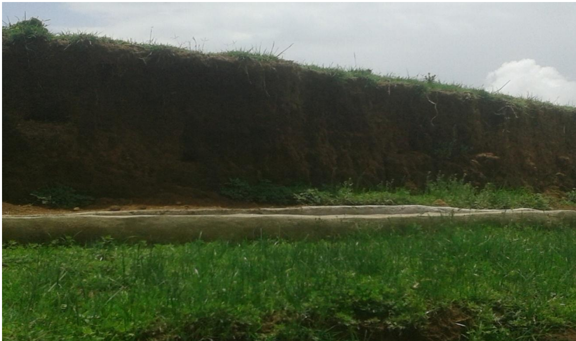
Figure: 4. 6Problems of erosion at the canal (tankua)
