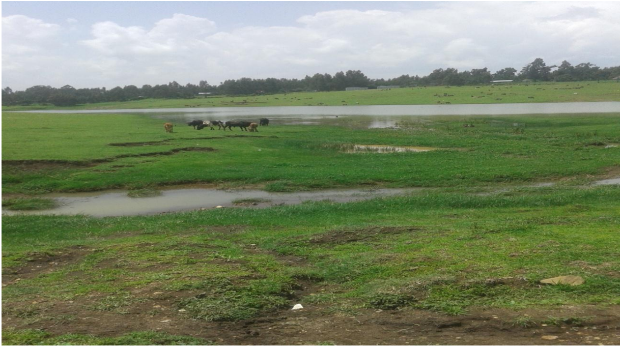
Figure: 4. 5Problems of erosion at the dam (Kuhar)
