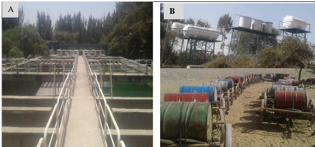
Figure 2.4: (A) Ziway water supply treatment plant (not functional at present); (B) Functional fluoride treatment plant using aluminum sulfate (Tejitu village)
