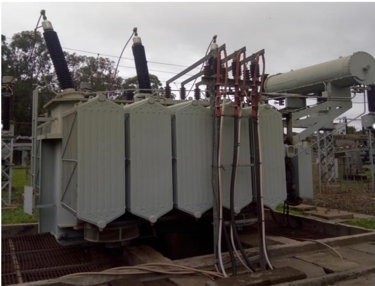
Figure 3. 1 Wolaita Sodo distribution substation 132/15 kV transformer
