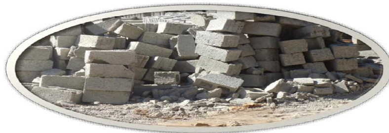
Figure2.5: Poor material handling [26].
