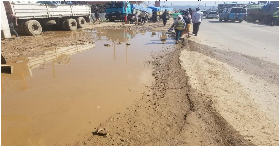
Figure 4. 14 Improper side and cross drainage at Kersa
