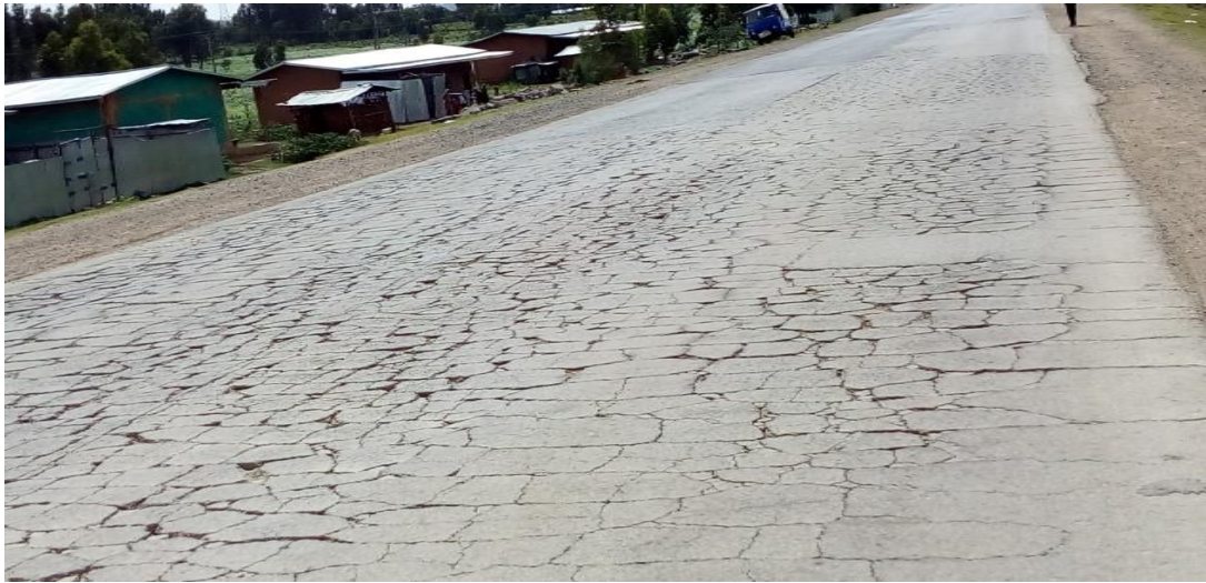
Figure 3. 6: High severity alligator cracking (June, 2018)
