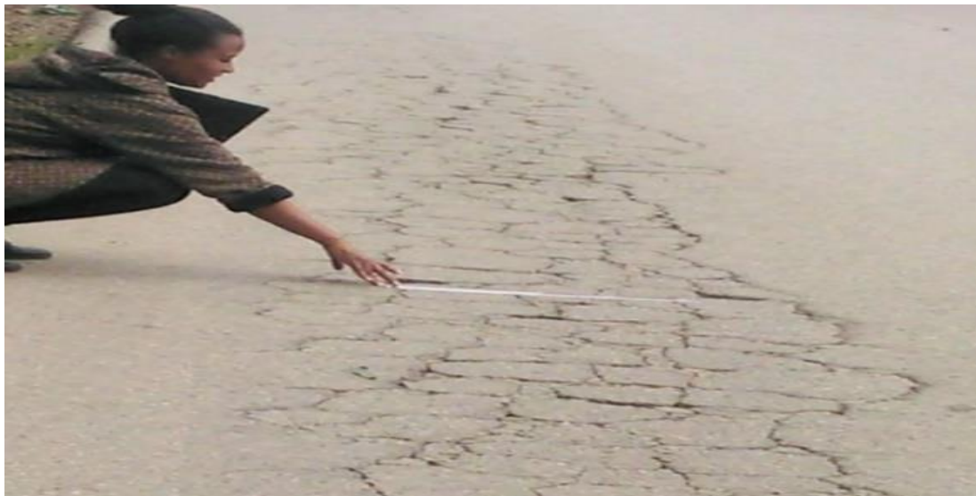
Figure 3. 5: Medium severity alligator cracking (by Tekalign Morka ,June, 2018)
