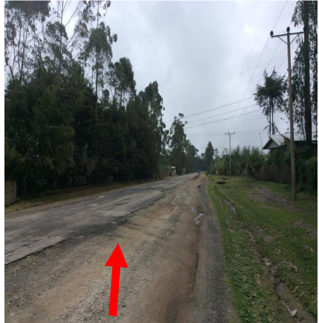
@ Doyogena Town to Hobichebe Pavement Carriageway totally Failure Coordinated (37.1895E, 7.317981N)
