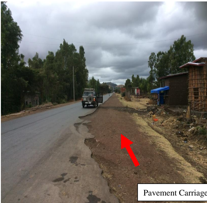
@ Butajira Town Pavement Carriageway Failure @ Coordinated (38.379035E,8.100408N)
