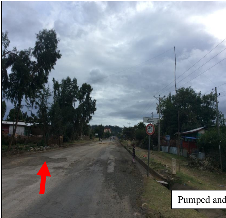
Fonka Town Pavement Carriageway Failure @ Coordinated (37.968852E, 7.7658579N)
