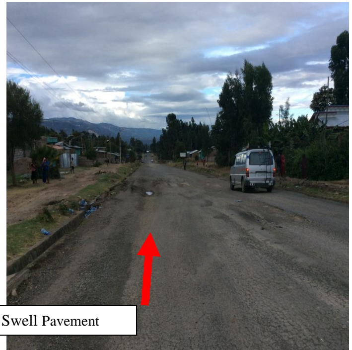
Fonka Town Pavement Carriageway Failure @ Coordinated (37.968566E, 7.655235N)
