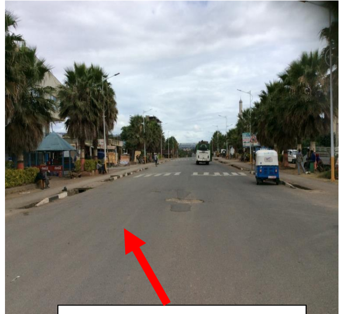
Carriageway and ditch Failure
