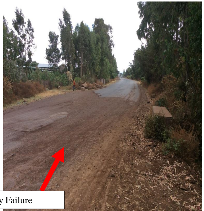
@ Butajira Town End Pavement Carriageway Failure
