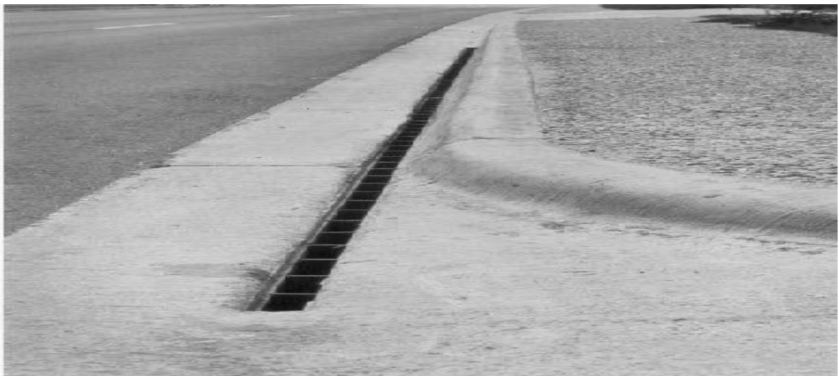
Figure 2.4 Slotted drain inlet at an intersection [23].
