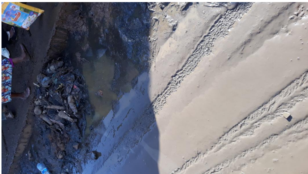
Figure 4.4 waste disposal on the drainage structure
