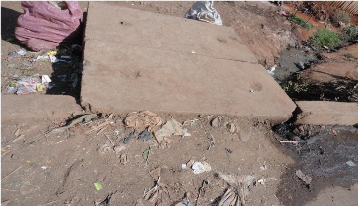
Figure 4.5 shows inlets closed by debris ( source: field survey ).
