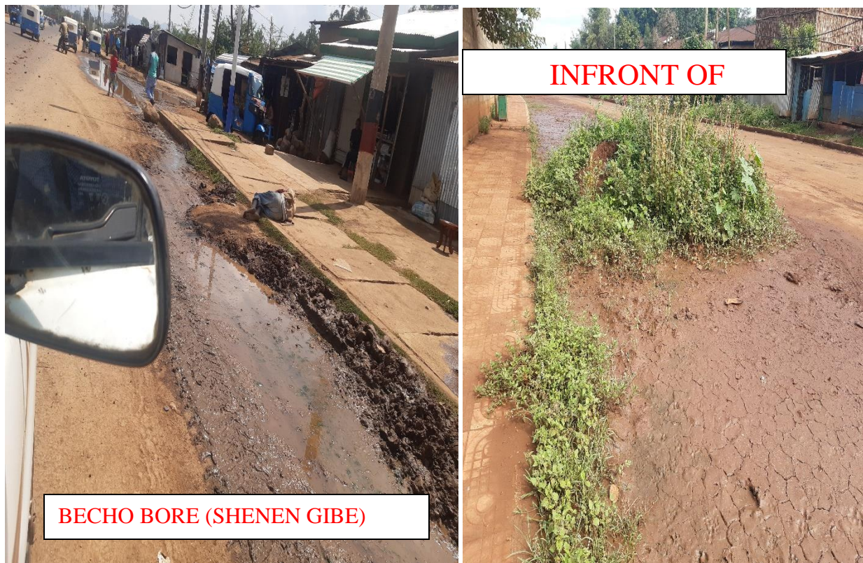
Figure 12. Sedimentation occurred due non accumulation of drainage and slope problem
