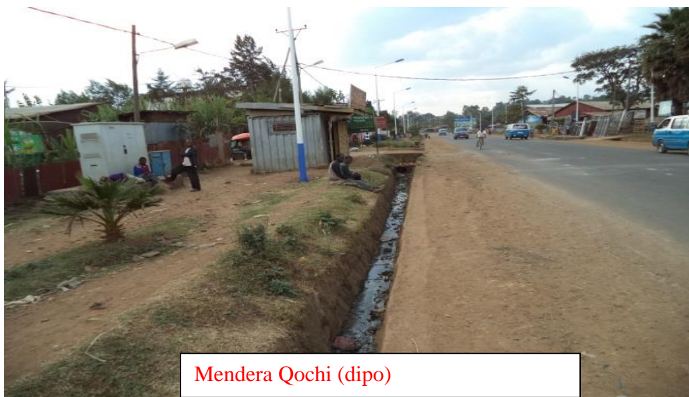
Figure 7. Channels which do not have silt trapping structures
