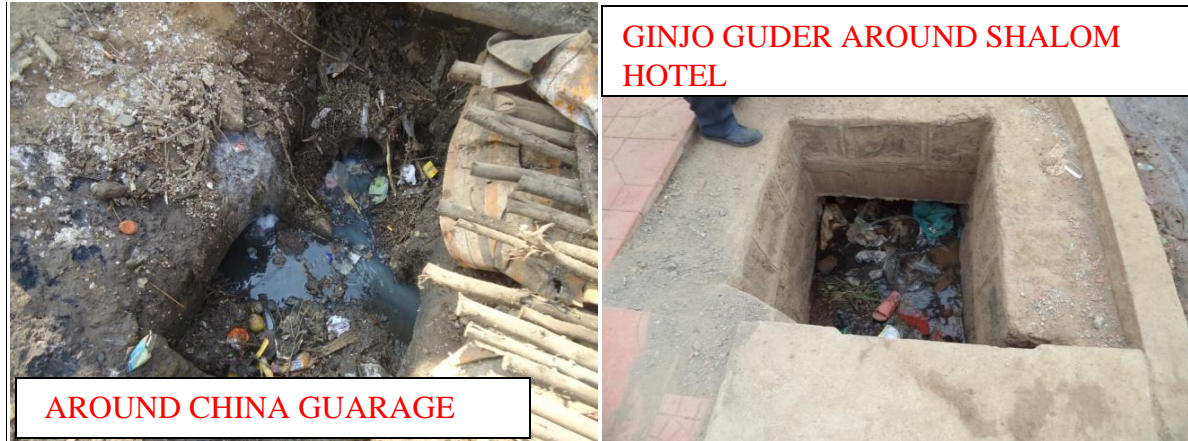
Figure 8. Disposal of solid waste into the storm water drainage channels and manholes
