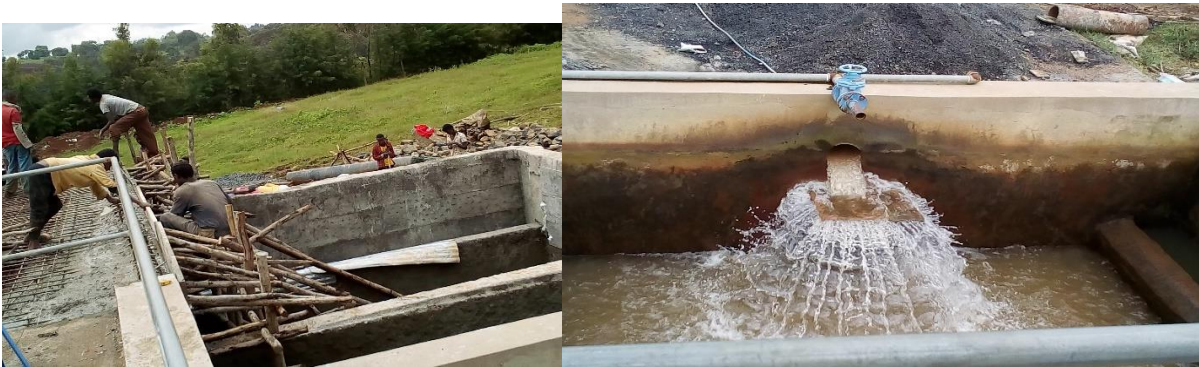
Figure N-2: Filter tank under expansion (left) and RSF (right)
