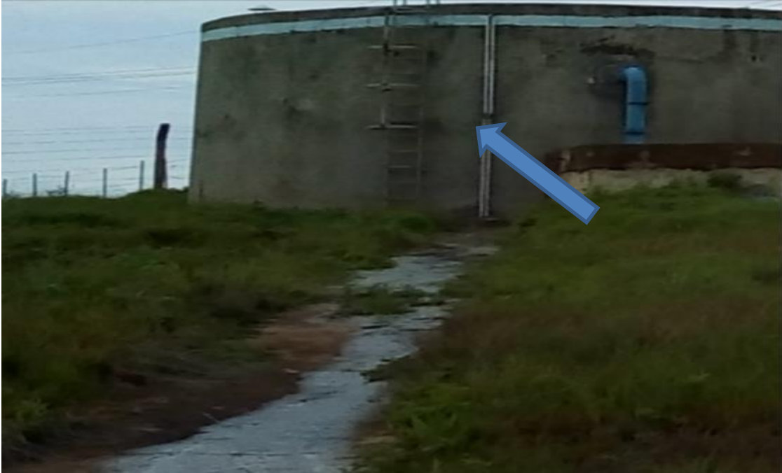
Figure 4.14: Leakage (Source: field observation, August, 2019)
