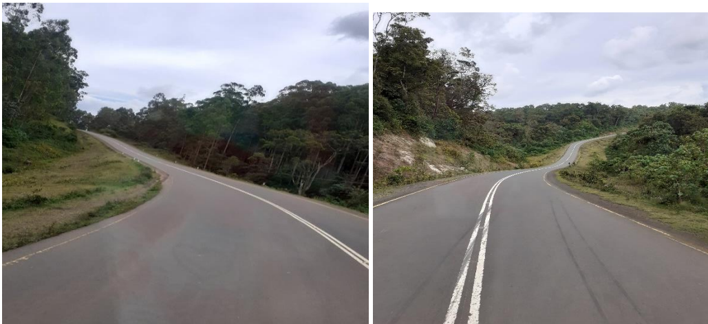
Figure 4. 14: Identified Blackspot in 460 at 25+80 (Source: Adinew G/michael).
