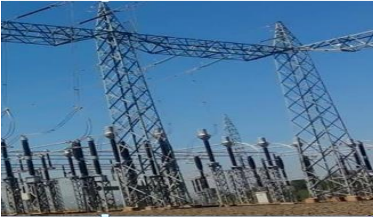
Figure5. 11 Partial view for Jimma substation
