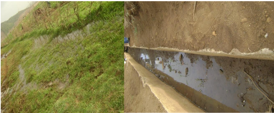
Figure4. 22 canal condition of Chena irrigation project
