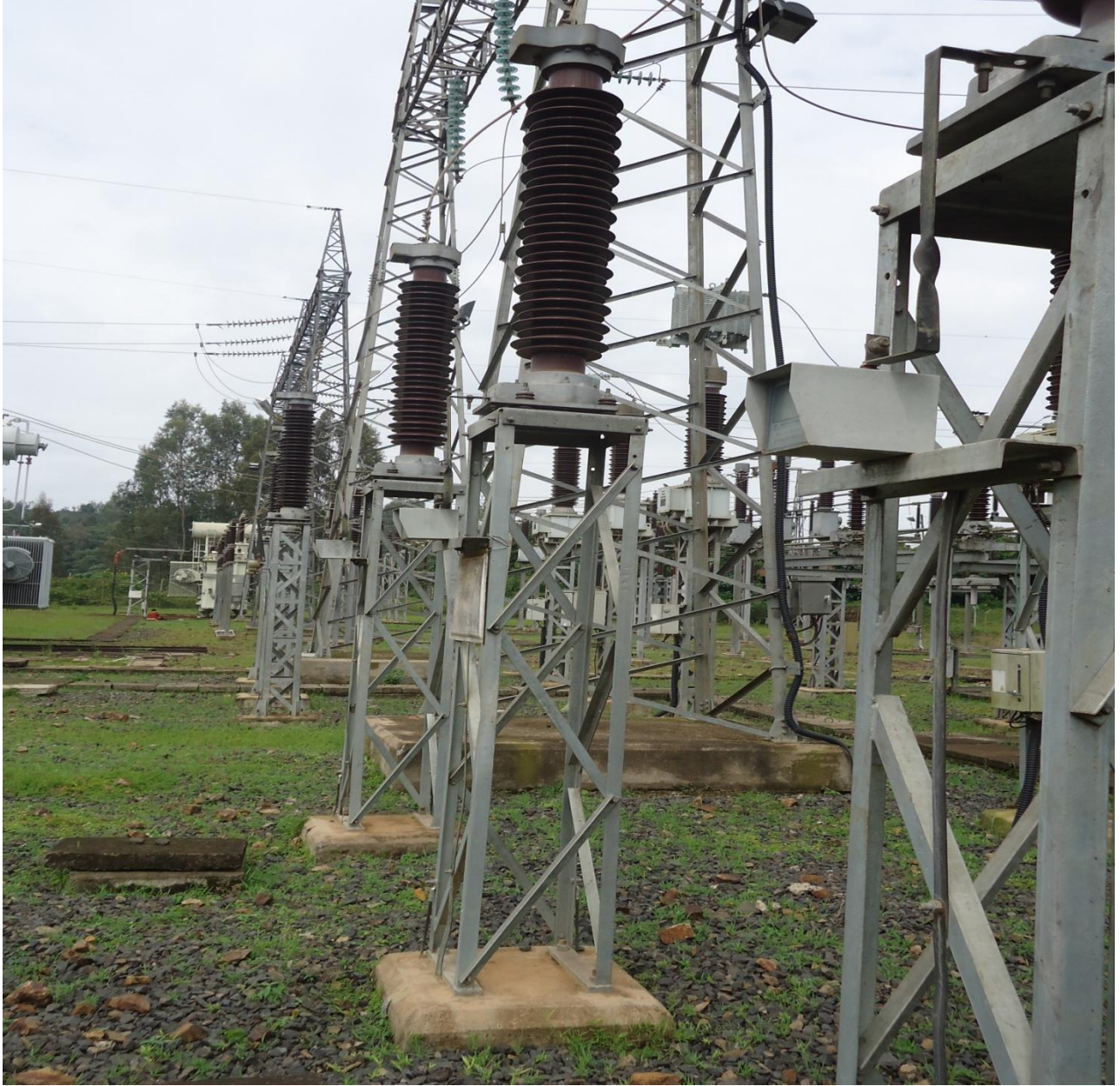
Figure 1.2 View of Jimma substation
