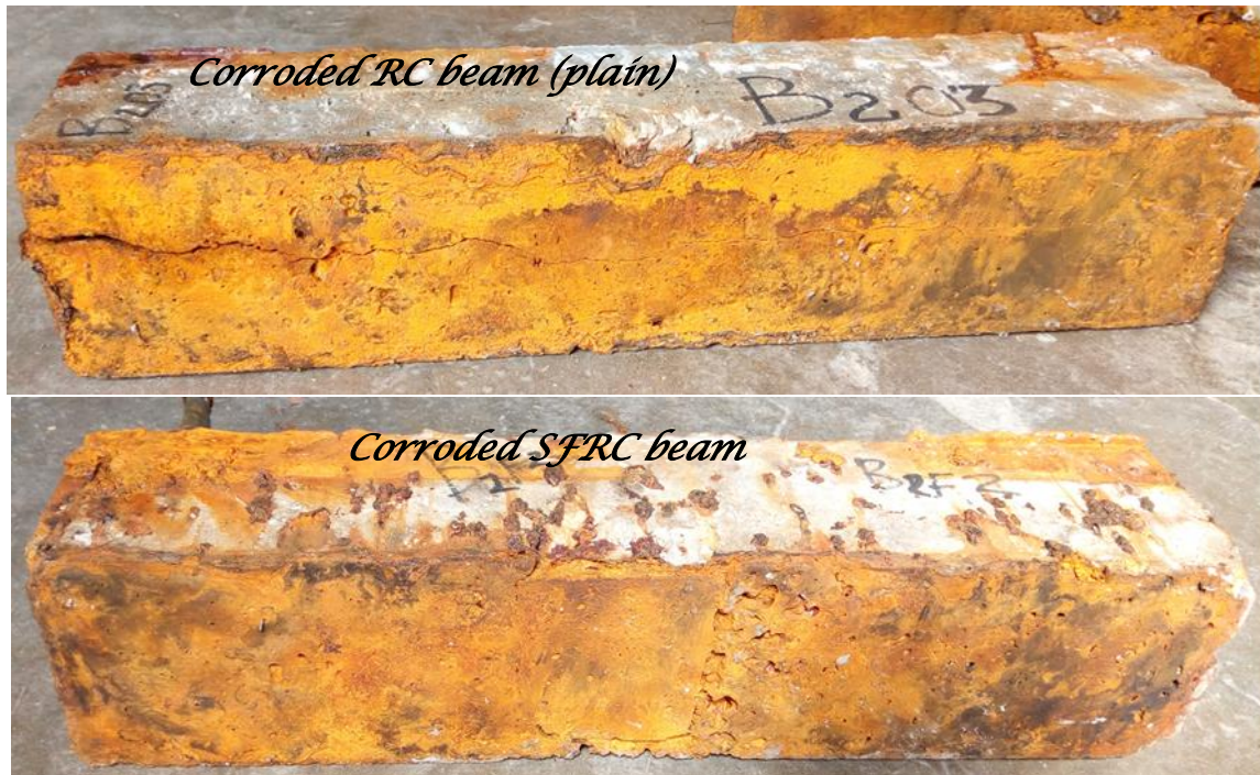
Figure 4. 18: Comparison between corroded RC (plain) beam and corroded SFRC beam
