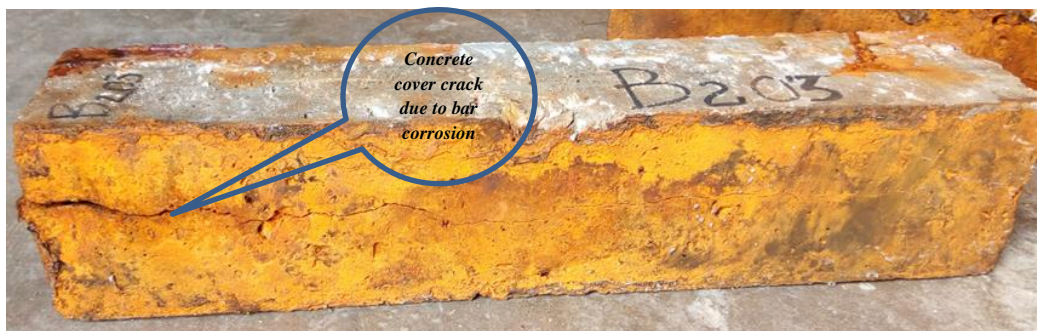
Figure 4. 17: Cracked RC beam due to corrosion
