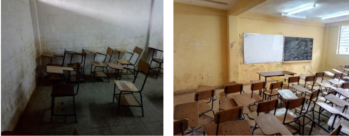
Picture 3: Class room shows lack of wall cleaning and needs painting in Mizan Tepi and Bonga Universities.
