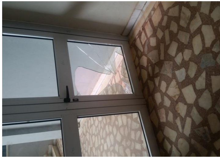
Picture 4 Broken doors which is not good for safety and appearance
