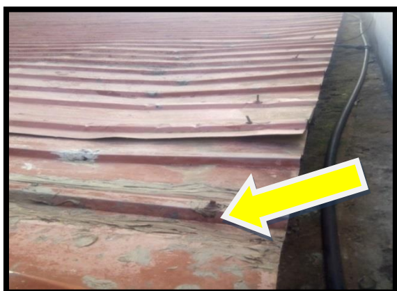
Figure 4. 11: defective roof tiles
