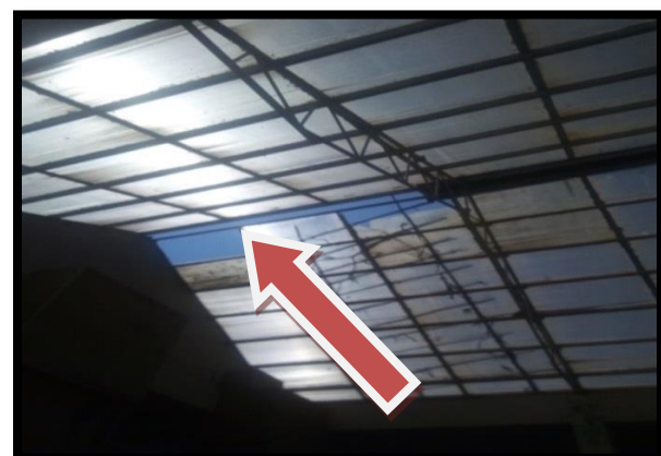
Figure 4. 12: Broken roof of skylight
