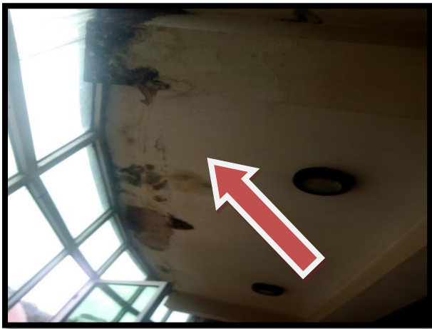
Figure 4. 9:- water seepage through top window window
