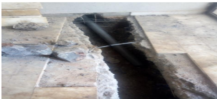
Figure 4.18: Faulty drainage wastewater
