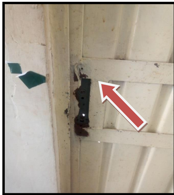
Figure 4. 8:- Handling damaged of metal door
