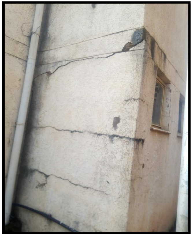
Figure 4.20:- cracking in exterior wall
