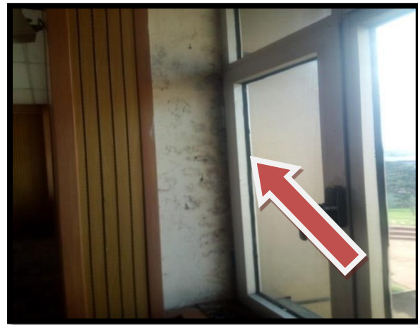
Figure 4. 10:- water seepage through side window
