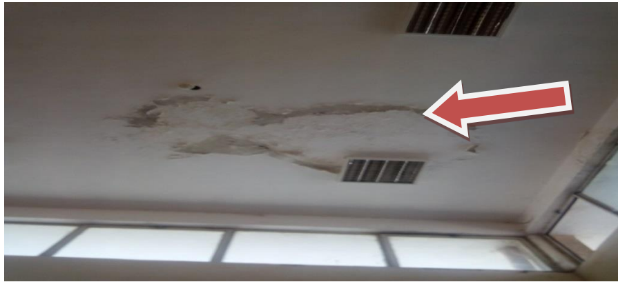
Figure 4.13: Leakage in flat roof
