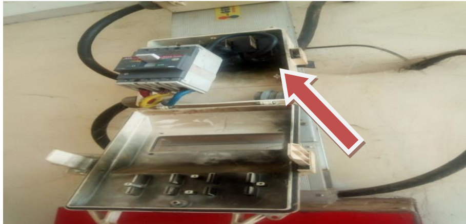
Figure 4.15: Short of circuit Breaker
