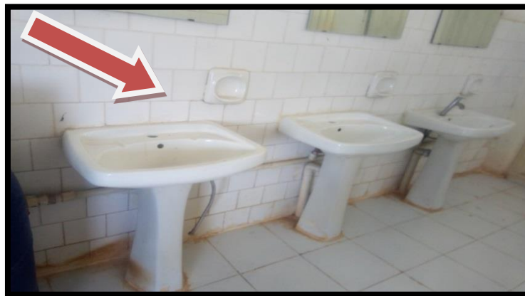
Figure 4.14: Sanitary accessories broken
