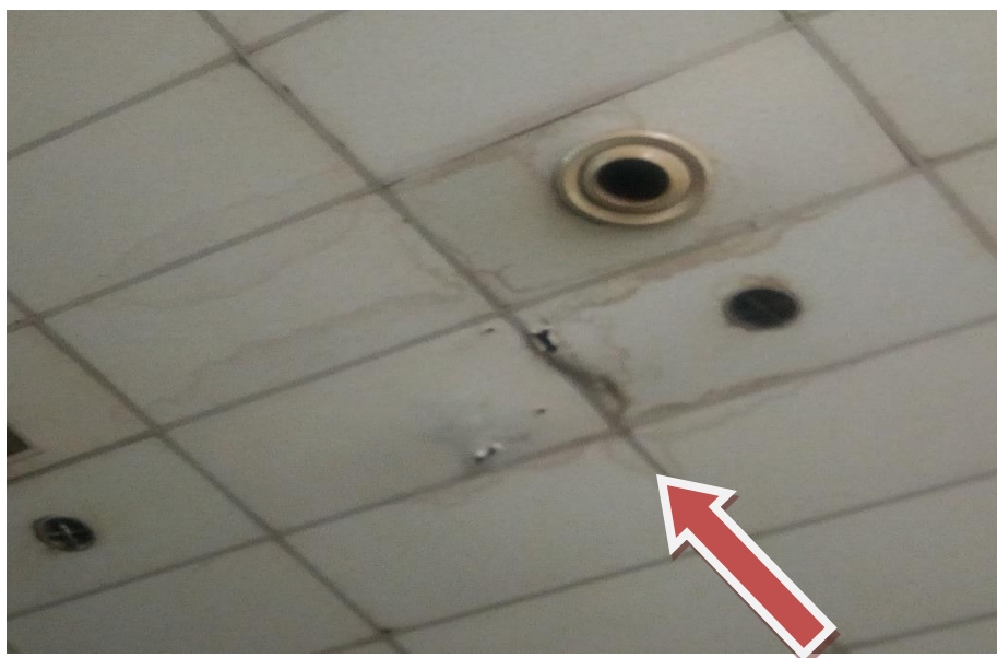
Figure 4. 6 : Leakages in ceilings
