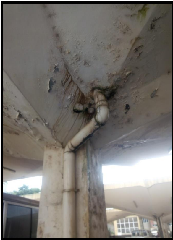
Figure 4.19:- downpipe leak in roof
