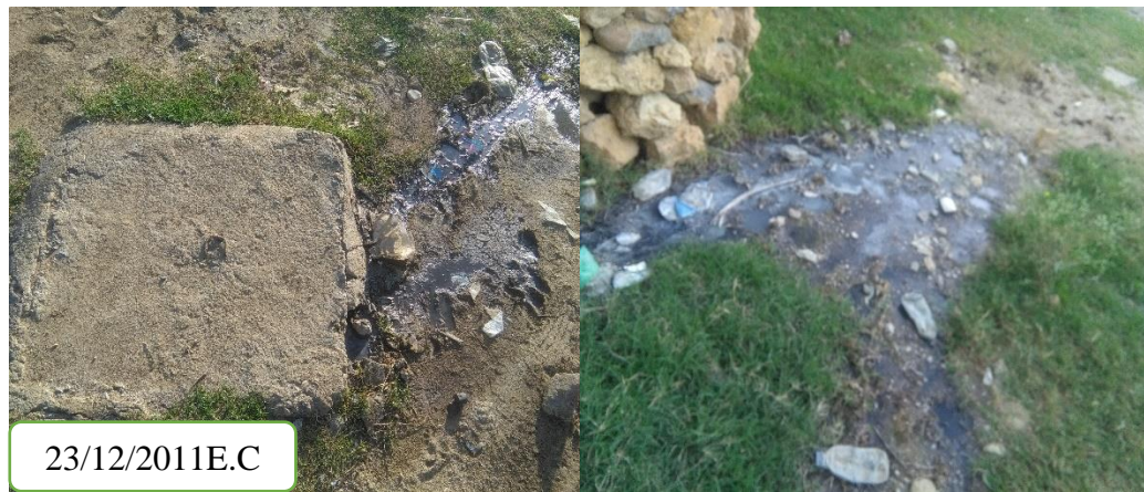
Figure 4.5 Septic tank leakage in Senet condominium
