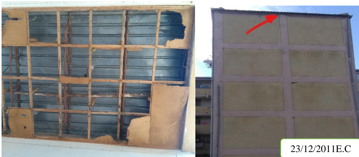
Figure 4.4 Roof defect in Edaga Bieray condominium
