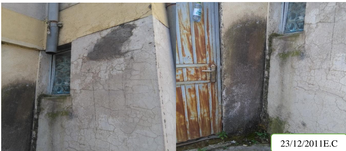
Figure 4.7 Condominium dampness in Edaga Bieray
