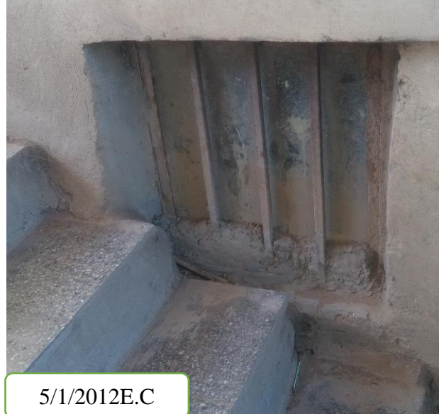
Figure 4.11 Design deficiency in toilet window
