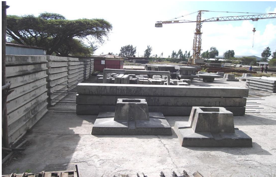
Figure 4.8: Fixed crane at precast production factory
