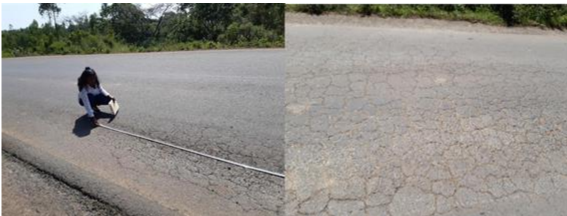
Figure 3.3: Longitudinal and Alligator Crack
