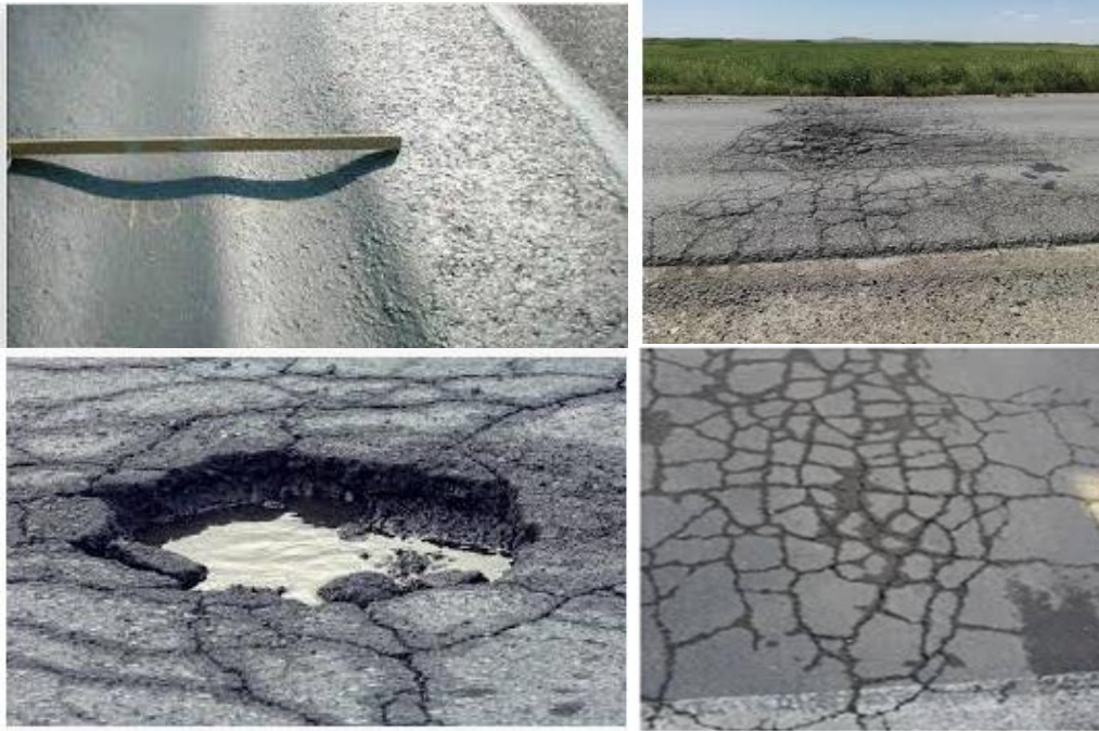
Figure 2.2 Flexible pavement distress [14]
