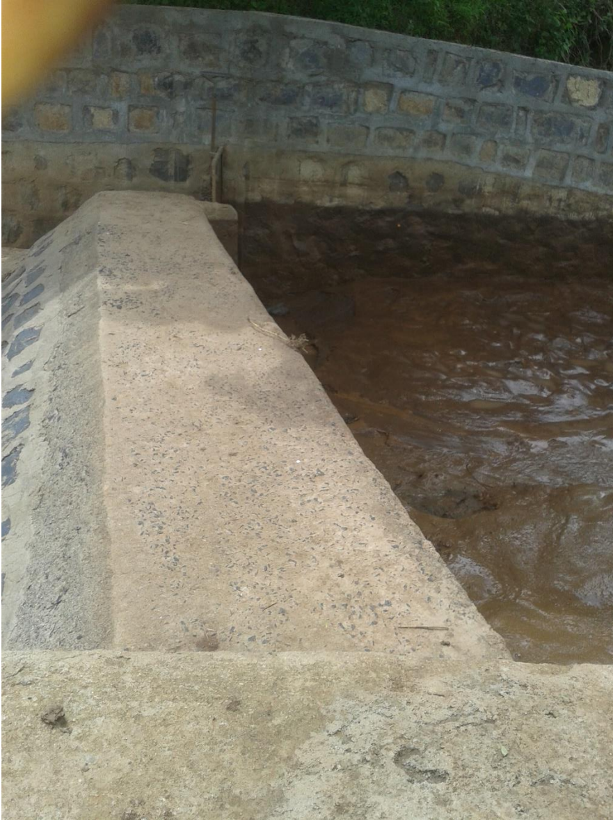
Appendix Figure 5. Silt deposited at u/s of the weir
