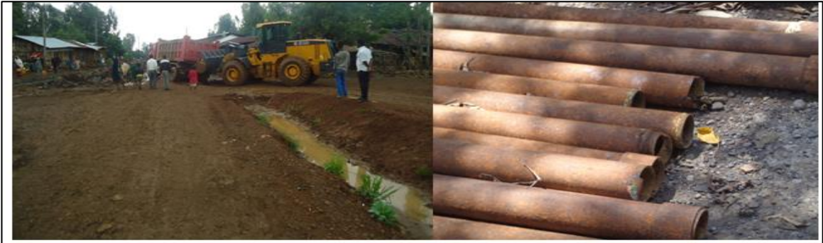
Breakage of pipe during road expansion
