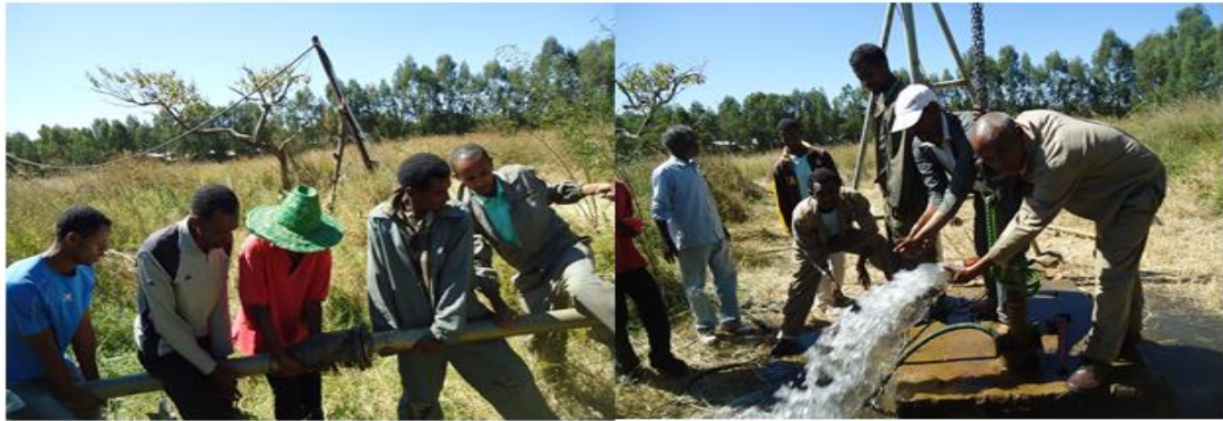
Breakage of pipe near to source
