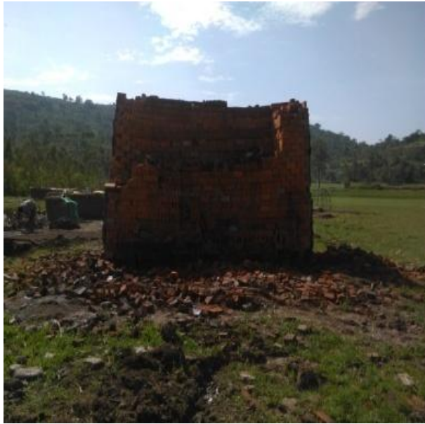
Photo-13 Broken bricks in Askola bricks production kilns
