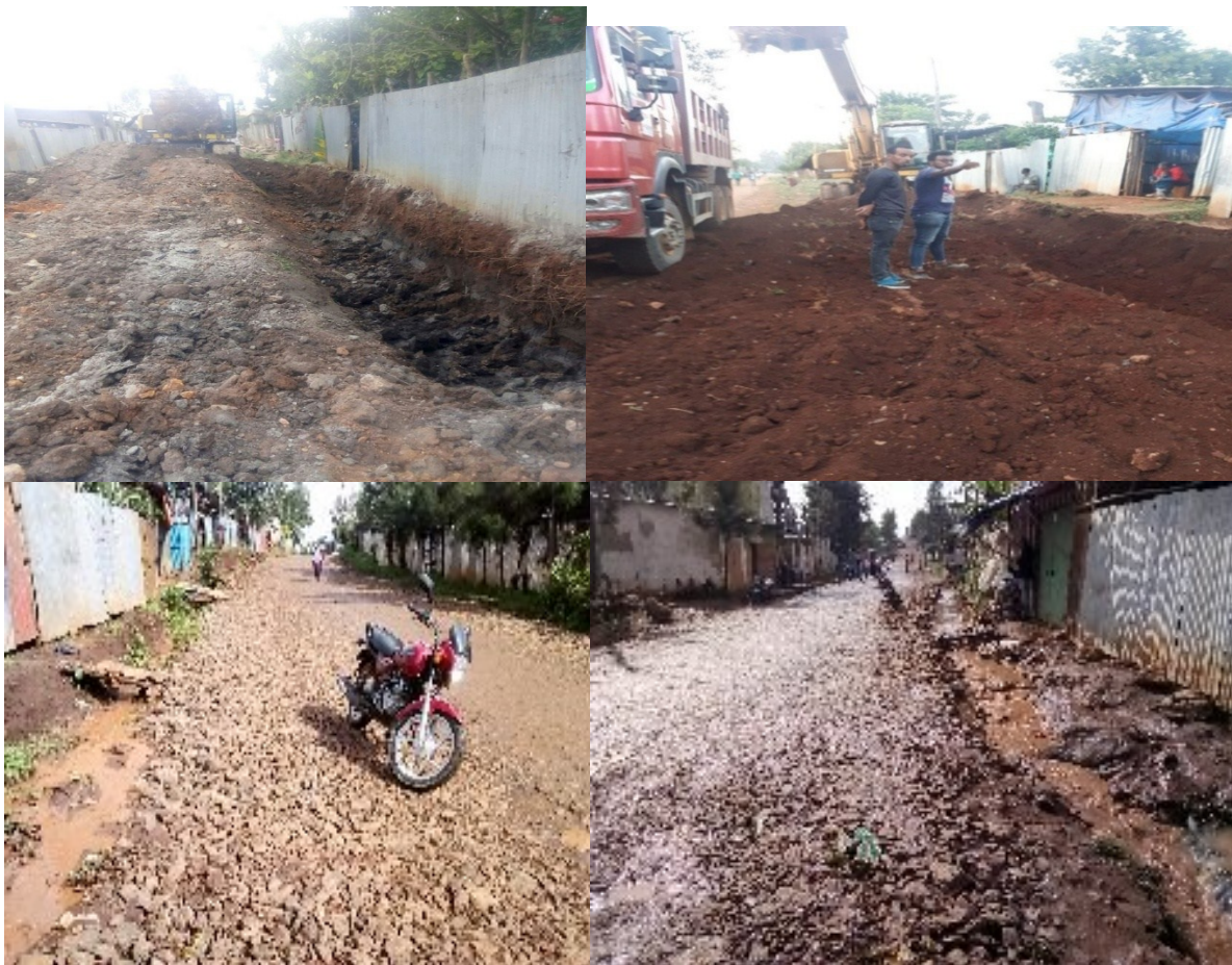
Figure 4.122 Roads with design problem.
