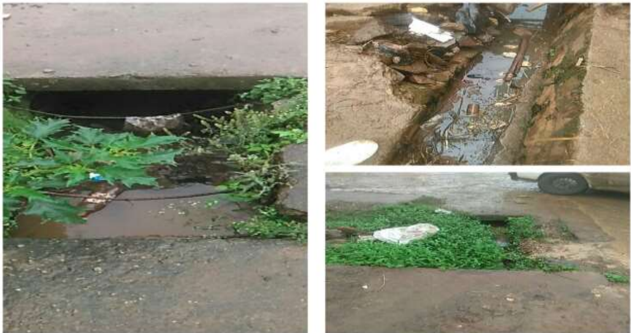
Figure 4.3: Damaged and sedimented ditches with poor existing drainage system at in front of bust station (photos on field, June 30/2021 at 11:00)
