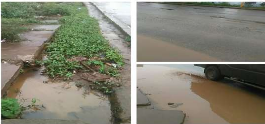
Figure 4.2: Effects of existing drainage system at in front of Bonga town municipality office (photos taken on field, June 29/2021 at 5:30)
