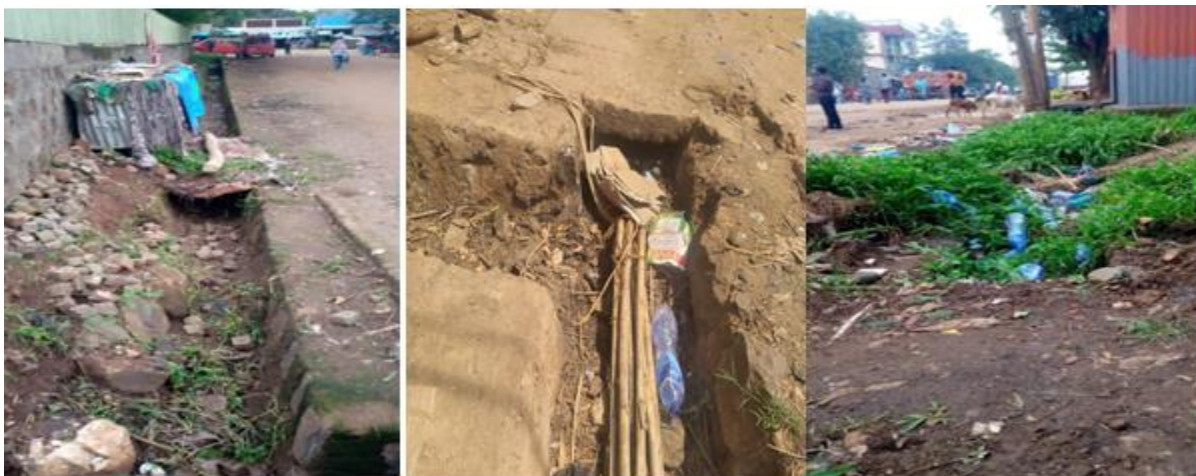
Figure 4. 14: Destroyed and detached, drainage structure
