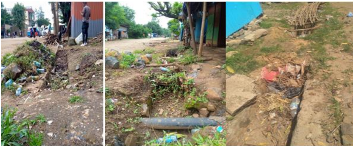
Figure 4. 12: Current Situation of Existing Drainage System in the Study Area
