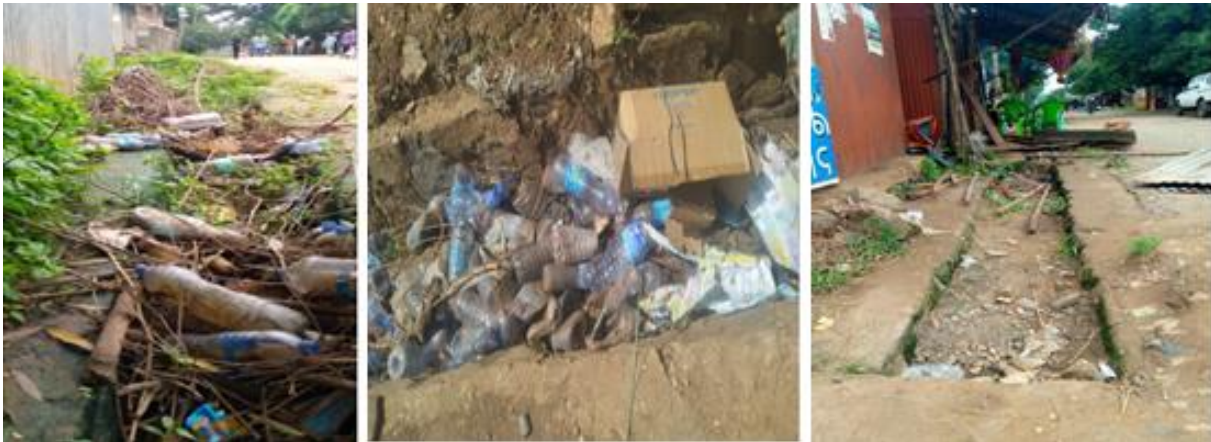
Figure 4. 13: Dumping of solid and liquid wastes in to storm water drainages
