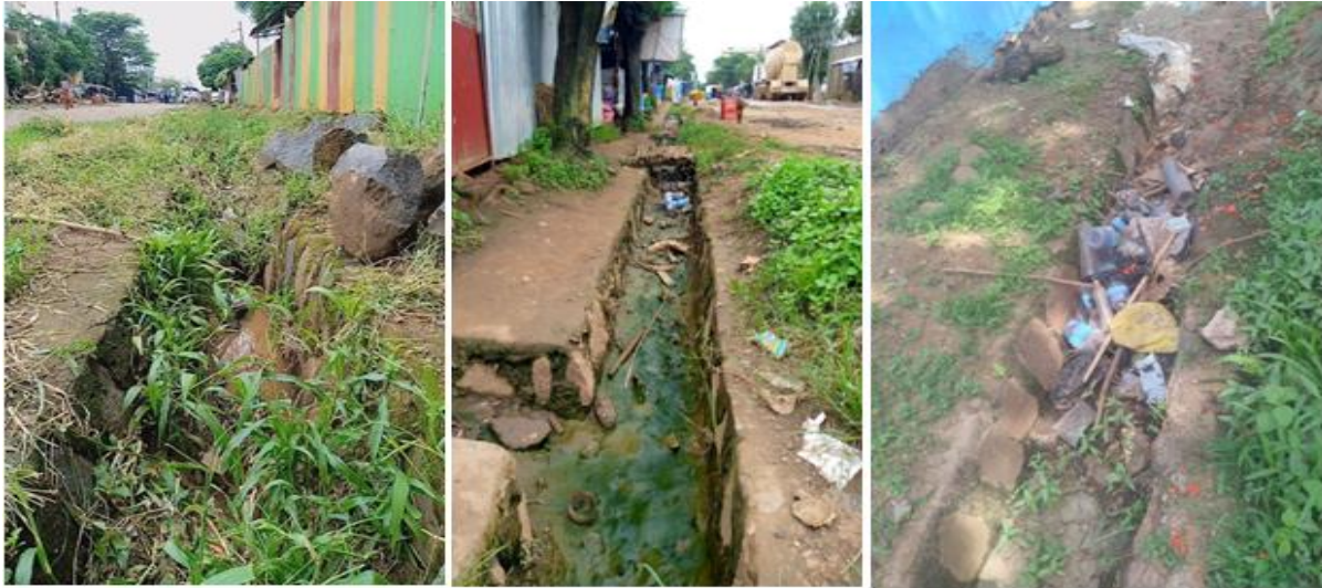
Figure 4. 15: Absence of regular clearance of drainage system
