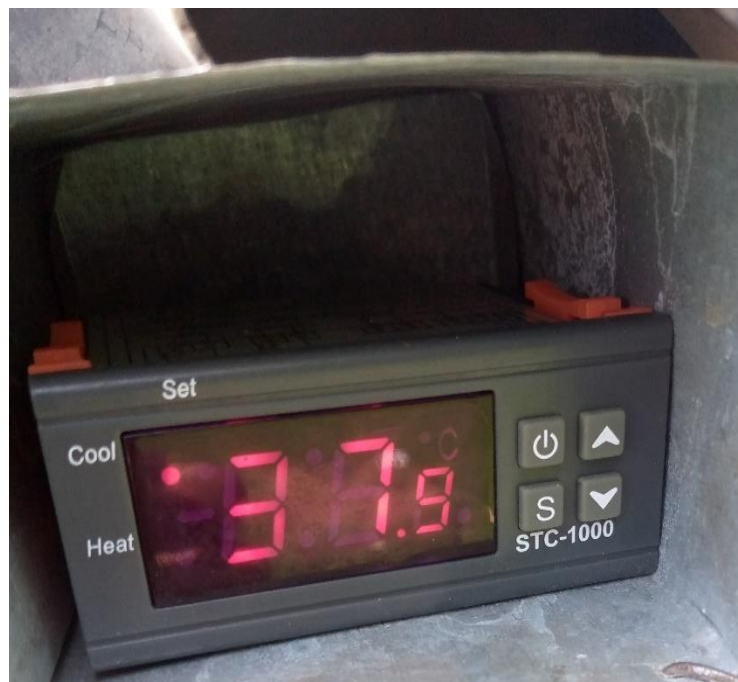
Figure 3. 8 Temperature controller device (Thermostat STC 1000)
