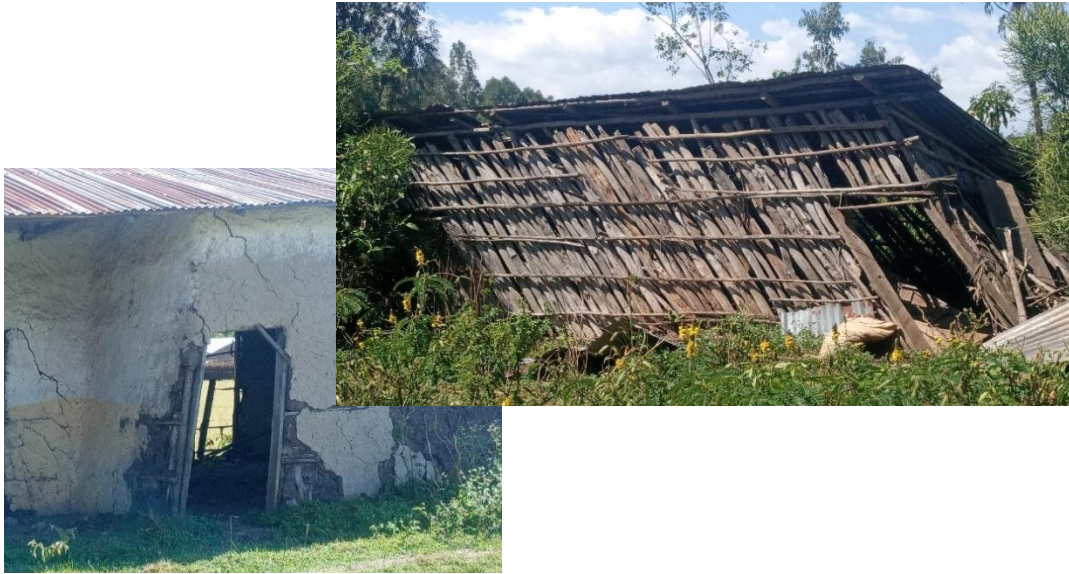
Figure 6: Relocates home collapsed due to bad soil type and window and door sold (Image taken: 15/06/2020 at 04:29 PM)
