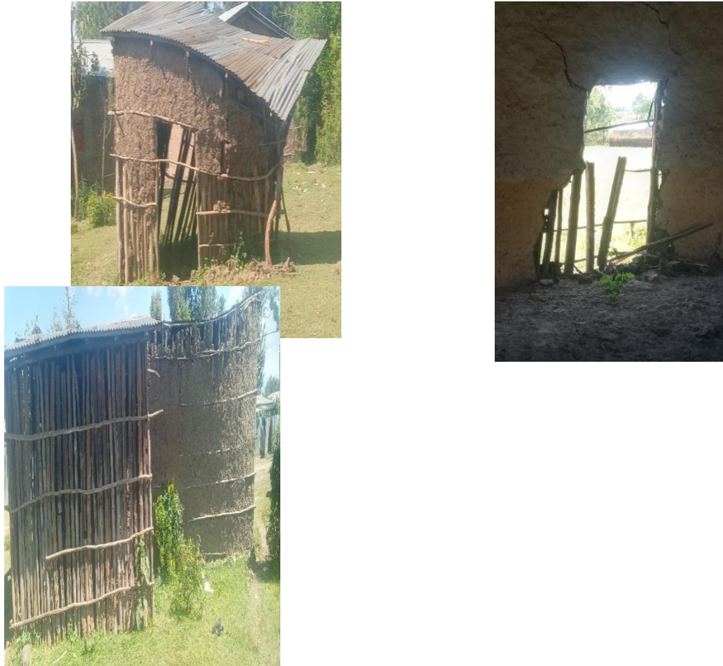
Figure 7: Relocates' poor housing condition and corrugated iron sheet sold (Image taken: 17/06/2020 at 09:15 AM)
