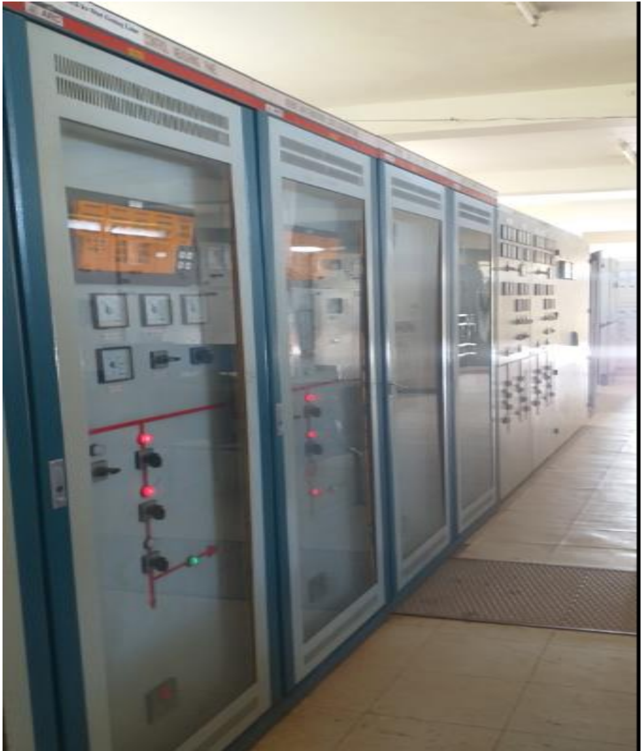
Figure 4.3: Oil circuit breakers and control room of Nekemte substation
