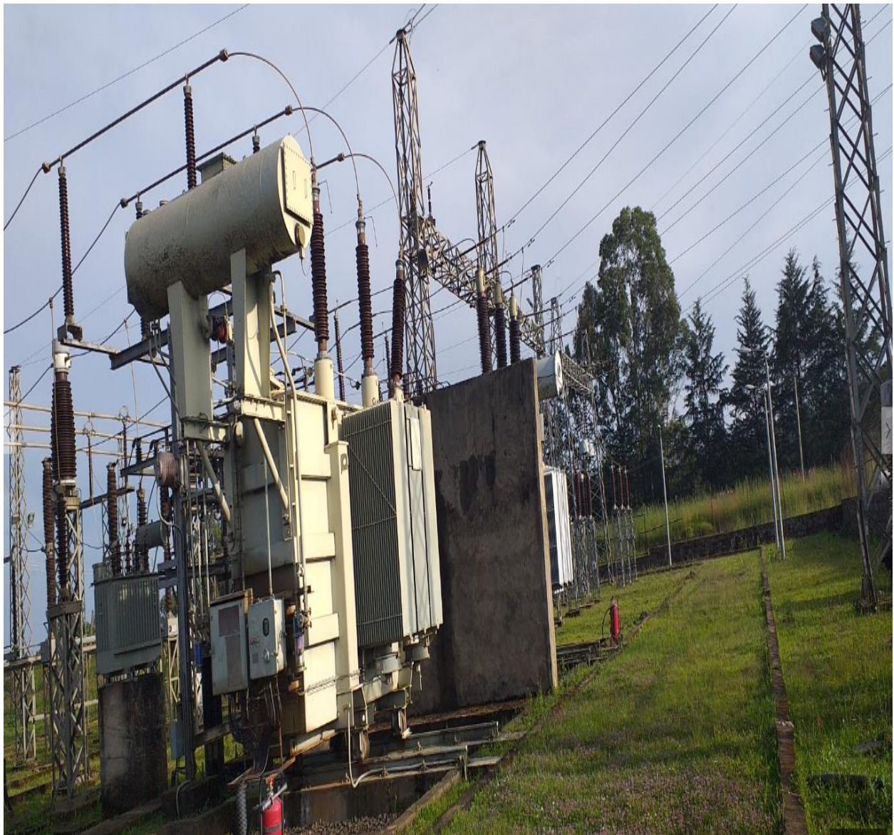
Figure 4.2: The general view of Nekemte substation taken during site visit
