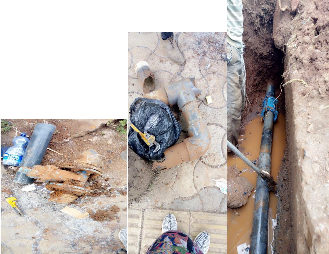
Figure 4 8: Breakage of pipe material and maintenance (9/2/2013E.C.)
