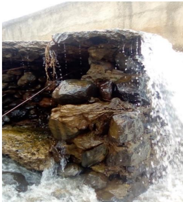
Figure 4. 9:- Improperly constructed downstream cut-off pile
