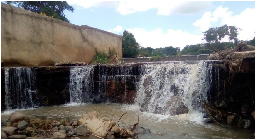
Figure 4. 10:- The effect of improper construction of pile structure.
