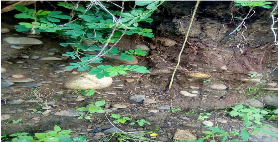
Figure 3. 3:- Right side river bank material.
