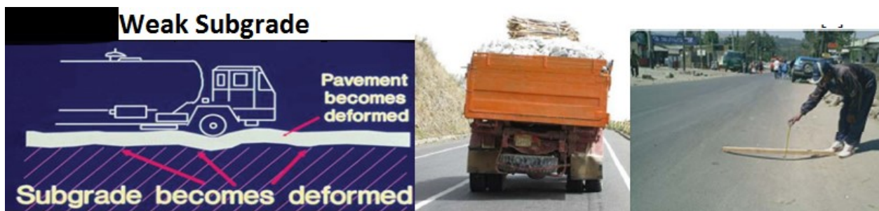
Figure 2.3: Pavement deformation due to weak subgrade [13]
