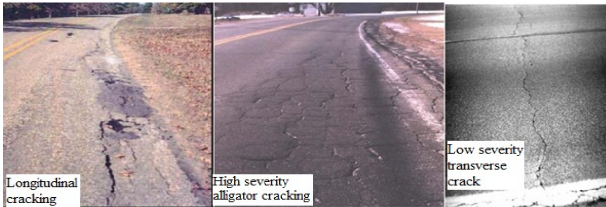
Figure 2.4: Pavement distresses because of expansive soil as road subgrade [3]
