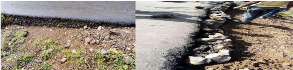
Figure 4.16 Observed problems on shoulder (By: Mengistu Bayu, 21th April, 2021 )
