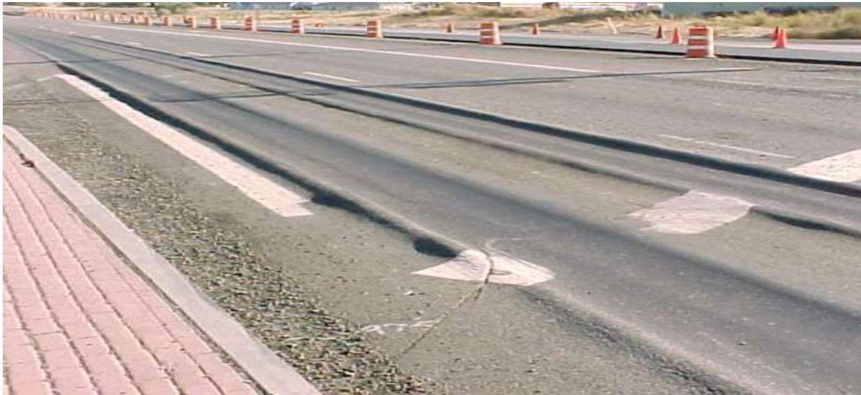
Figure 2.1: permanent deformation in Asphalt Pavement (Source: Google)
