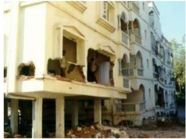
Figure 2. 4 Large scale damage in the upper floors (Murthy et.al. 2002)
