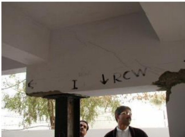
Figure 2. 3 Shear cracks in the cantilever stub beam supporting a floating column in a storey RC frame residential building in Ahmadabad. (Murthy et.al.2002)
