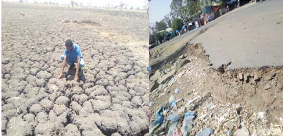
Figure 3-2 Visual investigation into expansive subgrade soils observed (April: 15/ 8/2013 3:45)
