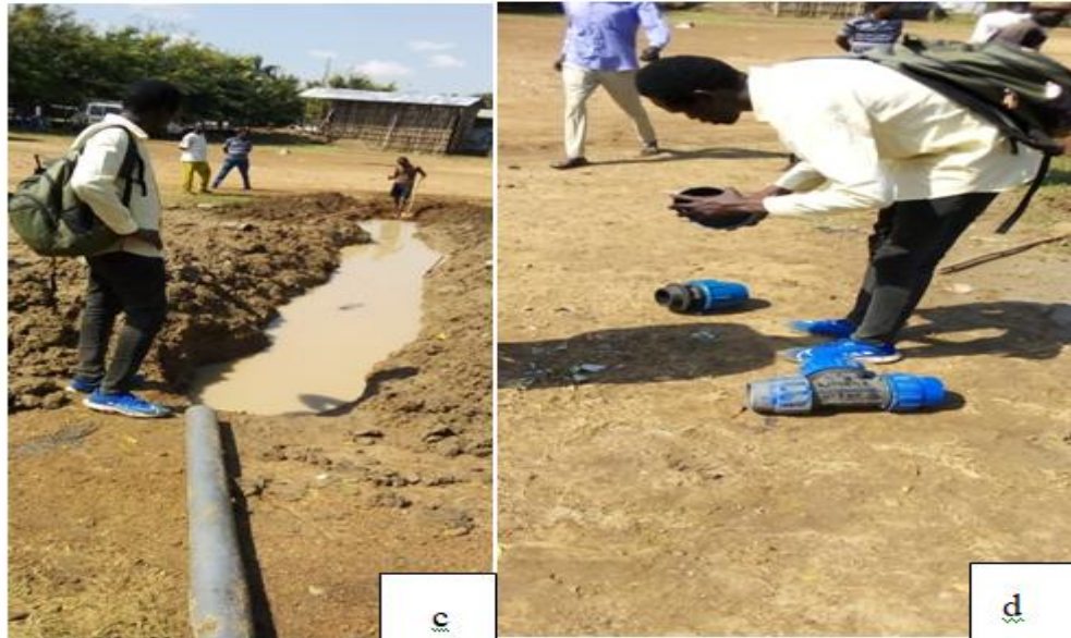
Figure 4.8: Photographs taken during Technical Investigation of Spare Parts in Kuergeng Town; c, Observing the broken Pipeline and d, Observing Spare Parts
