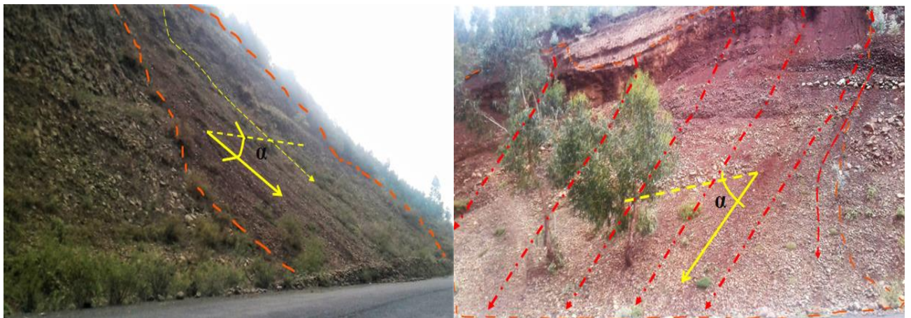
Figure 38. Sample photos that shows weathered rock-soil slope failure along road corridor
