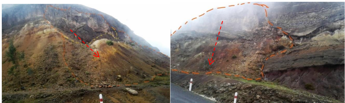
Figure 11. Sample photo that shows failure Rock-soil slope along road corridor
