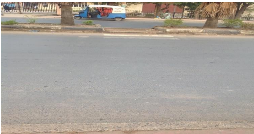
Figure 4.19: Lack of accessible curb ramp on either side of crosswalk
