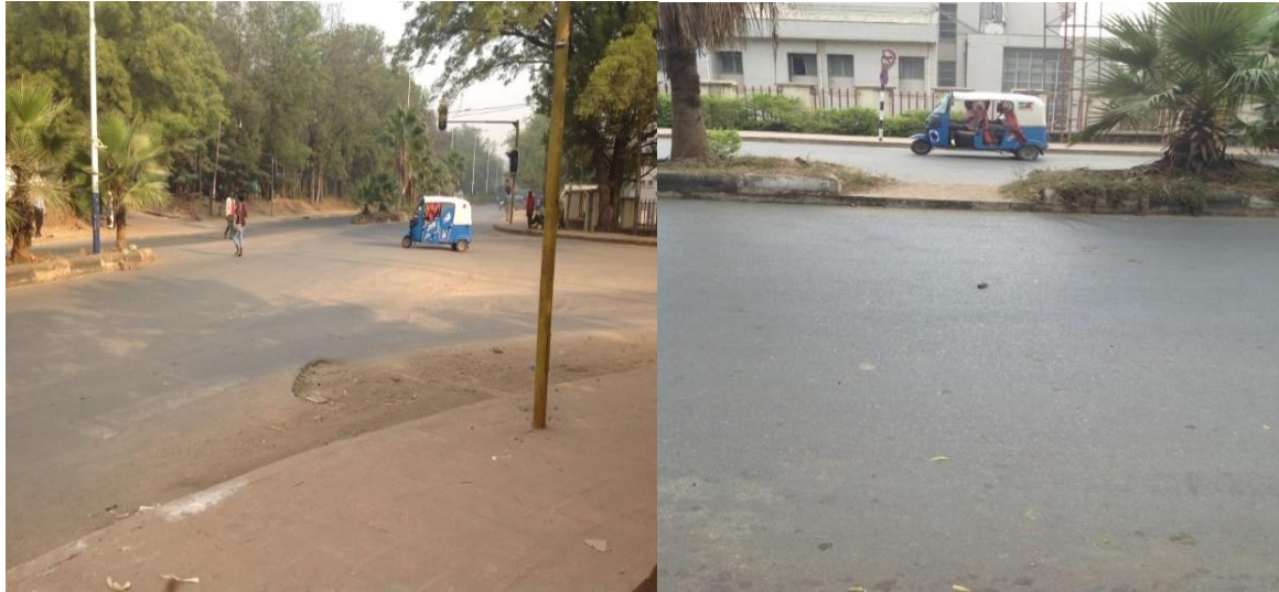
Figure 4.25: Lack of curb ramp and invisible zebra crossing marking
