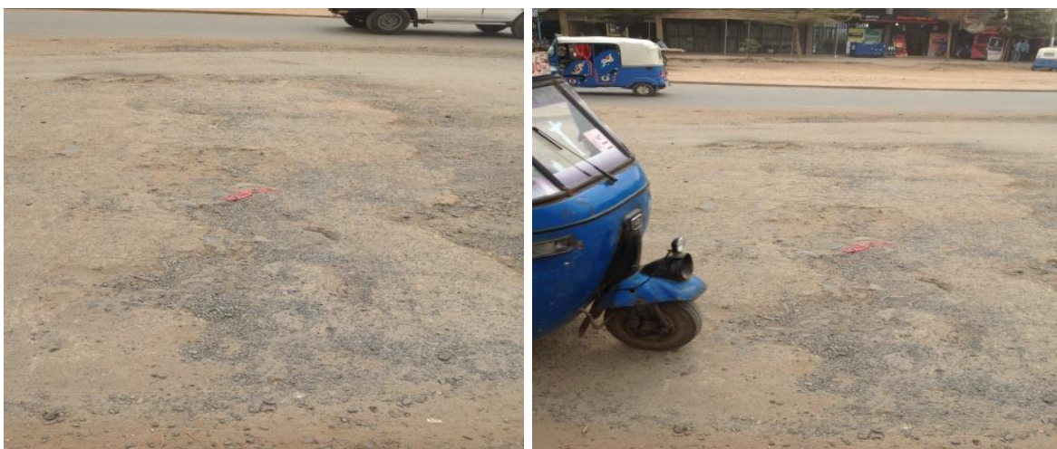
Figure 4.23: Poor crosswalk surface condition
