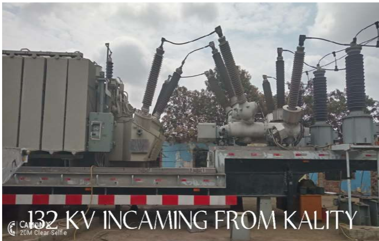
Figure 3.2 the 132KV in coming from Kality substation.
