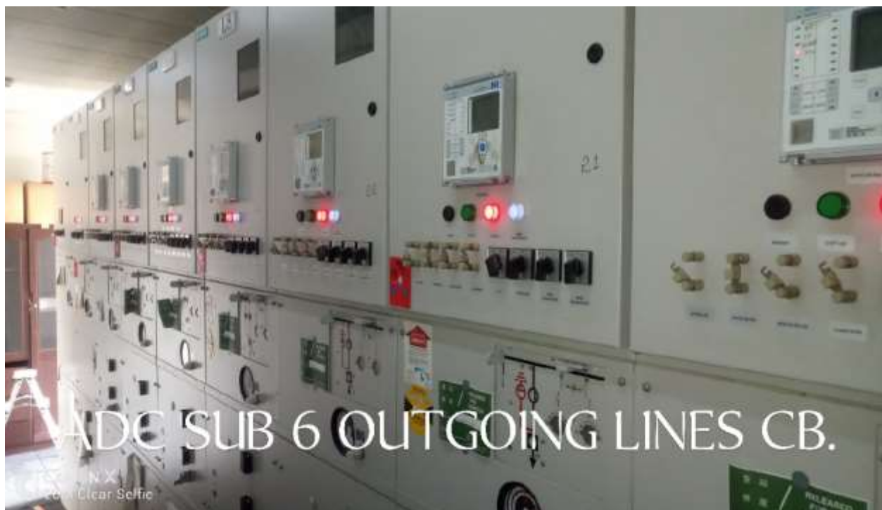
Figure 3.4 the Addis Center distribution substation 6 outgoing lines CBS.
