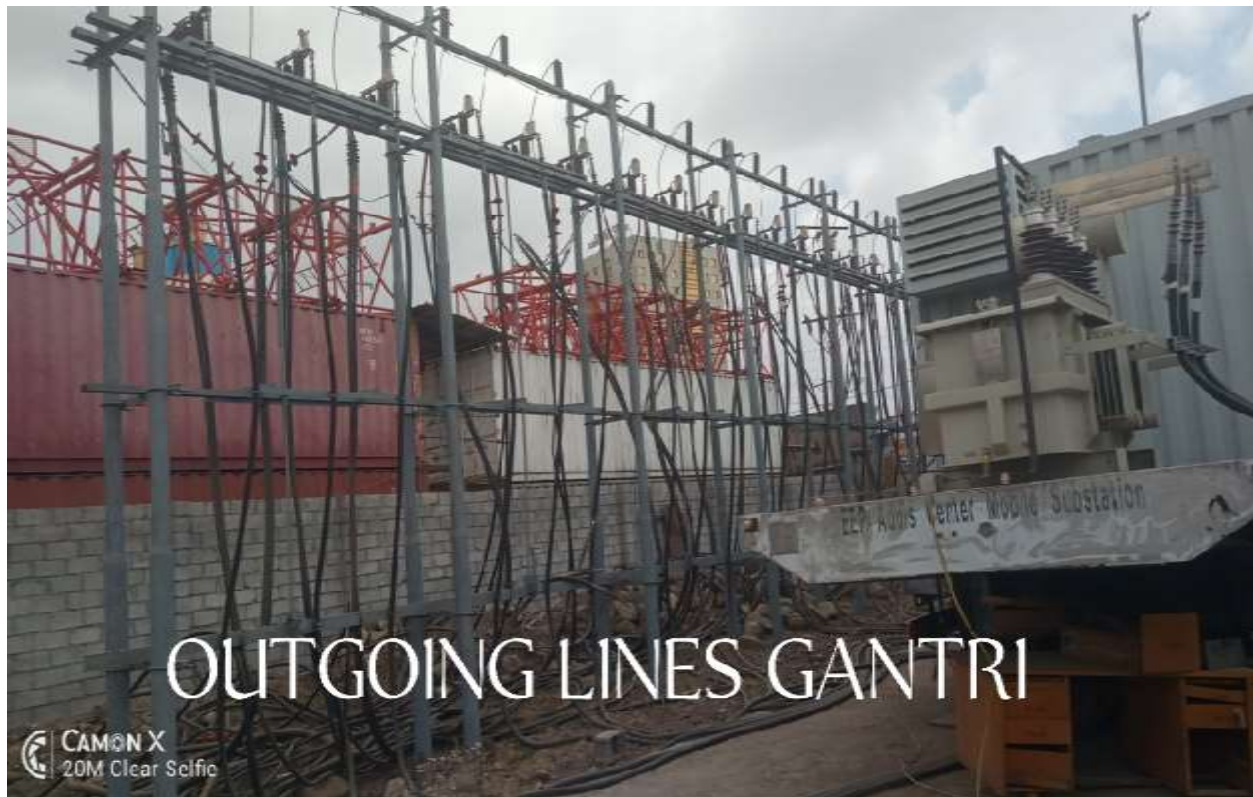
Figure 3.3 the Outgoing lines of Addis Center distribution substation.
