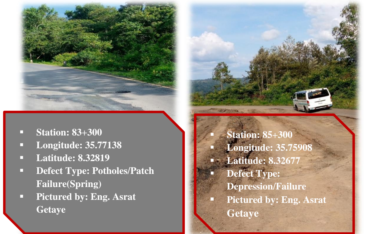
Figure 4.1: Selected road defects along Bedele – Metu upgrading road project
